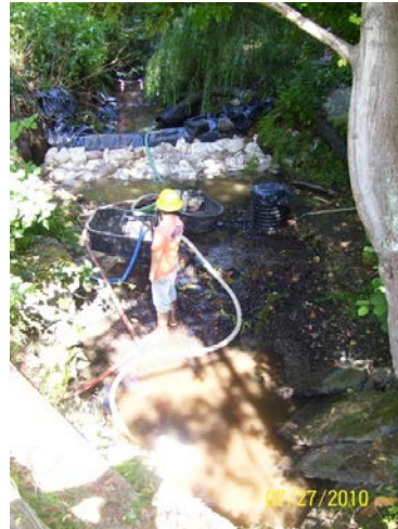
Figure 3-16 Stream Bypass Intake
