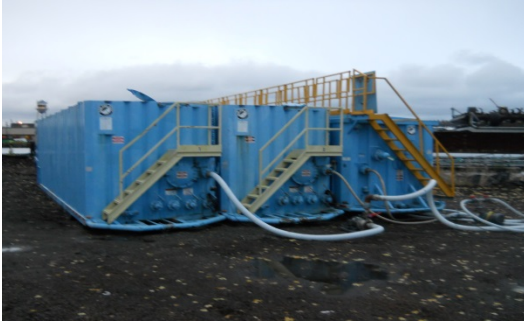
Figure 3-3 Settling Tanks Need Space
