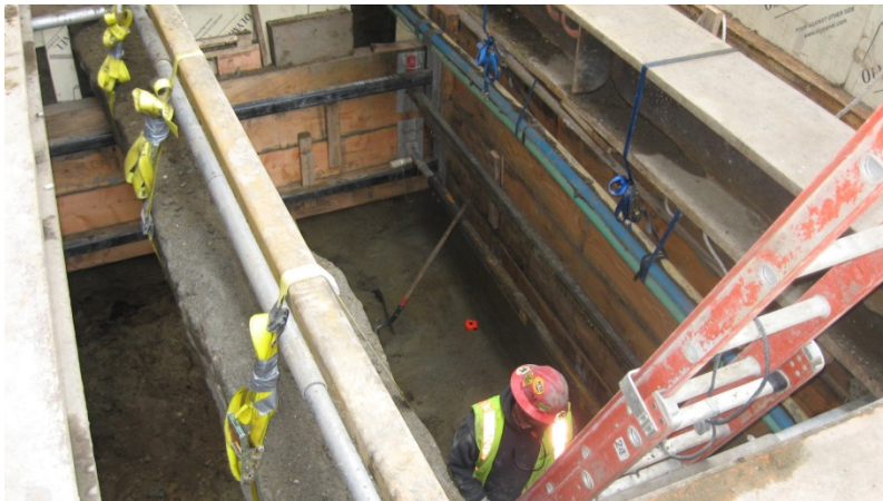
Figure 3-10 Beam and Strap Utility Support
