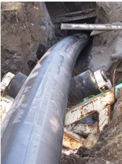
Figure 3-9 Damage and Danger to Conduit
