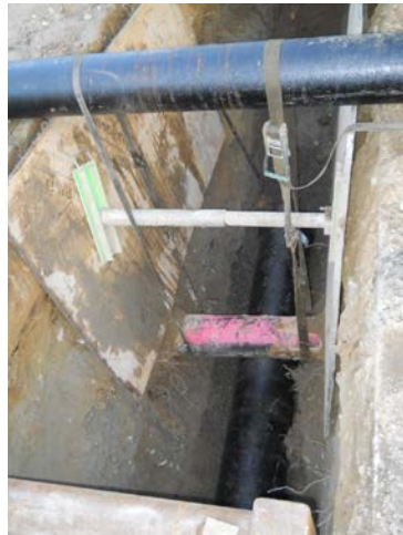
Figure 3-8 Water Main Supported with Nylon Strap
