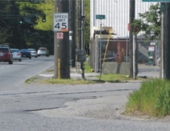
South segment has intermittent sidewalk on east side; walkways that exist have numerous obstacles.
