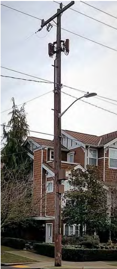
Typical wood pole design with panel antennas
