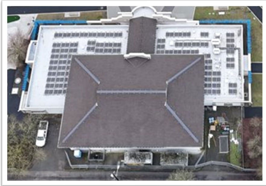
Aerial view of new solar panels at South Park Community Center, added to the renovation scope thanks to support from the Office of Sustainability and the Environment
