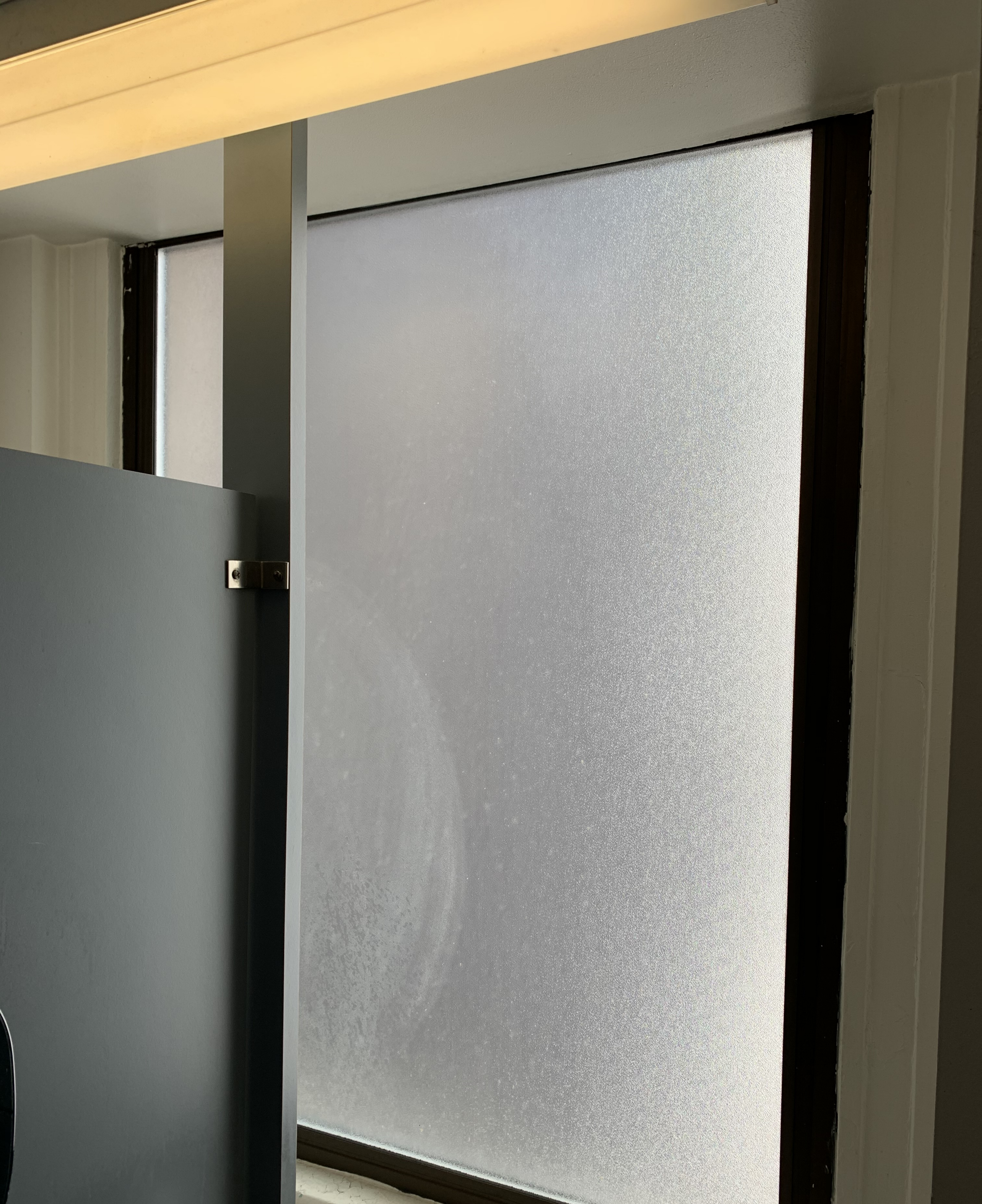
YWCA Interior - L7 - non-operable/obscured glazing window to be replaced - Alley October 2020
