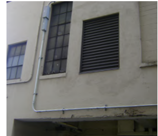
4 Exposed Non-Original Conduit and Mechanical Equipment Broken, Painted Windows
