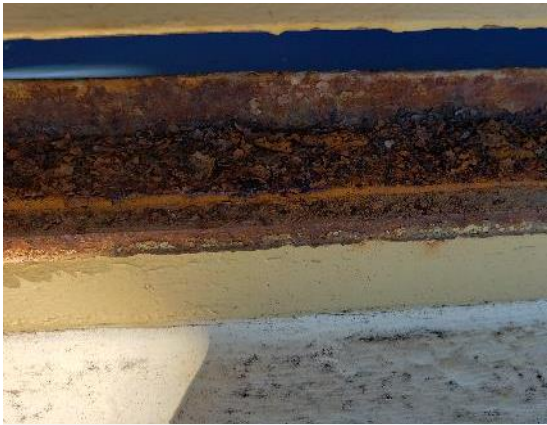
Rust scaling at frame beneath sash
