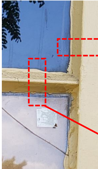
Photo above depicts the intersection of a steel muntin at a fixed window frame.
