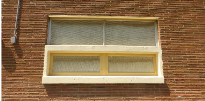
Narrow fixed windows below missing glass block walls
