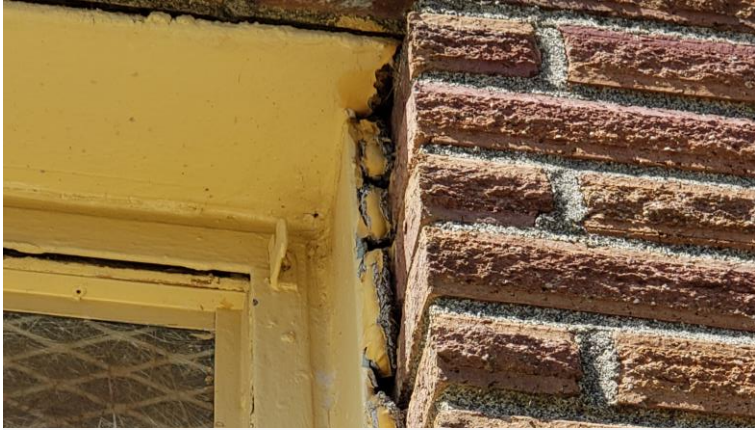
Failing asbestos sealant and steel angle corrosion
