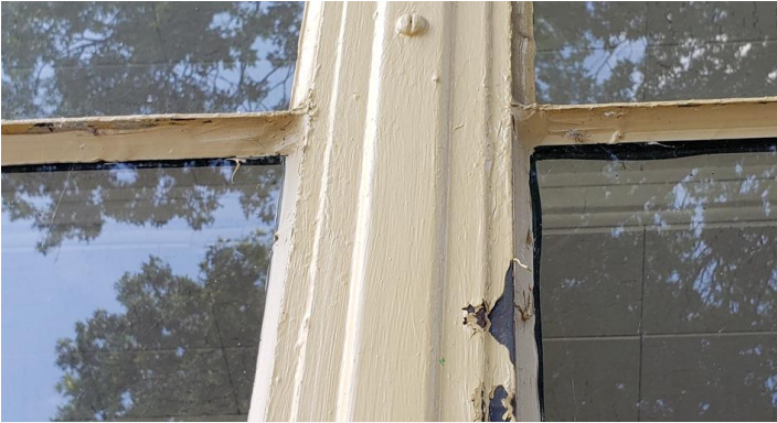
Corrosion at frame
