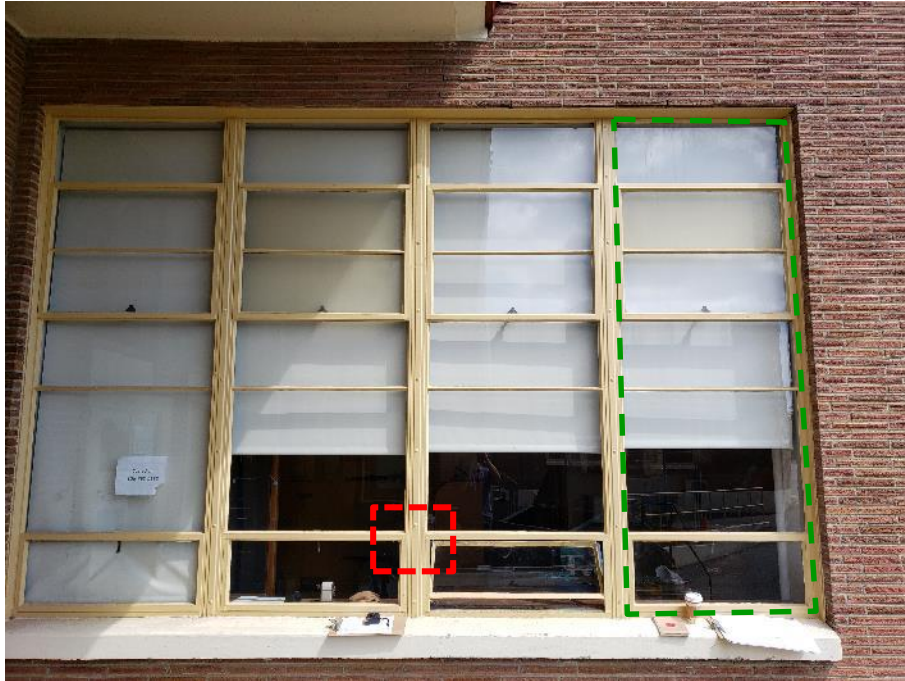
Photo above depicts four (4) office combination windows with the green dashed lines indicating the size of each window. The red dashed area indicates the location of the photo depicted on the right side of this page.
