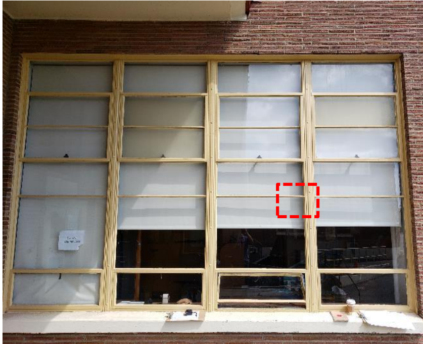
Photo above depicts the same four (4) previously shown office combination windows with the red dashed area indicating the location of the photos depicted on the right side of this page.
