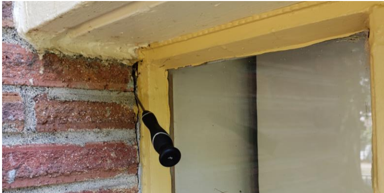
Window flange set against brick masonry without steel angle
