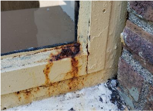
Corrosion at corner of sash and broken weld
