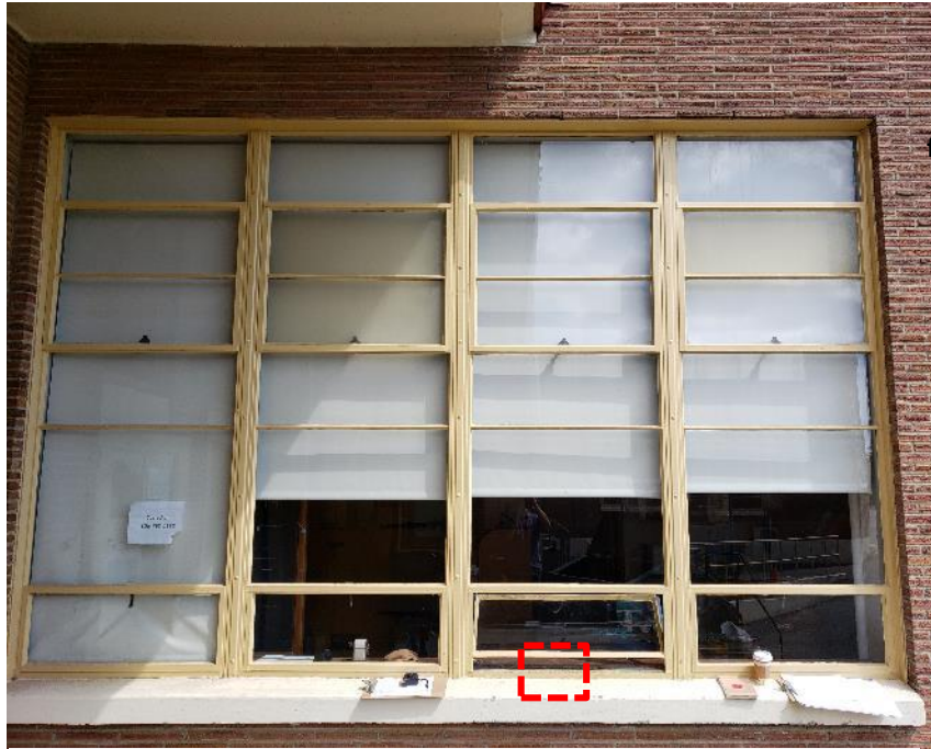
Red dashed area above indicates the location of the close-up photo shown to the right.
