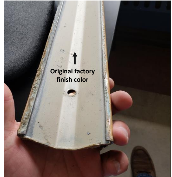
Photo above depicts the original smooth factory finish color on the back side of an interior steel mullion.
