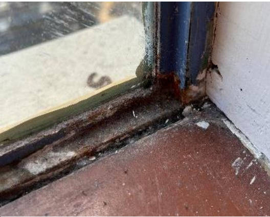
Rust scaling at interior of fixed frame
