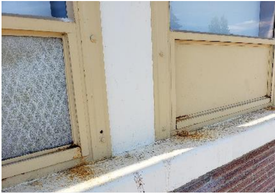
Corrosion at corners of sashes
