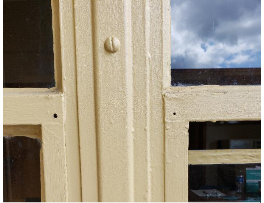
Close-up view of a typical painted steel mullion at the intersection of fixed and operable portions of the windows.
