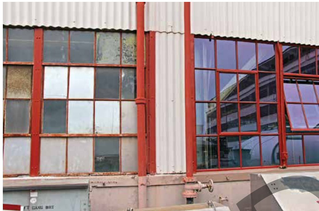
BEFORE and AFTER view of the Hope's Pearl Harbor Building 155 historic preservation project
