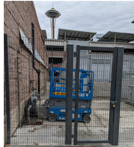
South Facade - existing gas equipment Shown dashed below
