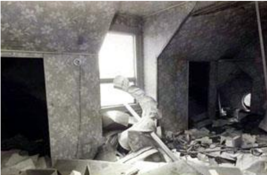
Figure 25. Bruce Lee's room during demolition. Note the same flower wallpaper. Photo courtesy of James DeMile.
