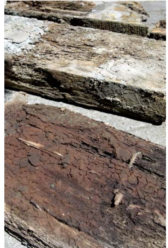
Gribbles—tiny marine wood-boring creatures—are damaging the seawall's wooden supports. Photo: Municipal Archives.
