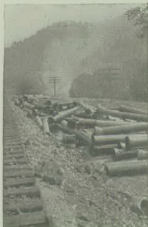
Pipe Improperly Unloaded
