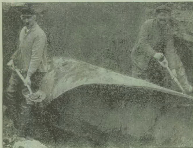
Large Rock Directly Under Break in Pipe
