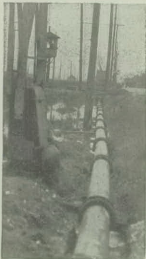
Dresser Type Couplings on Small Pipe
