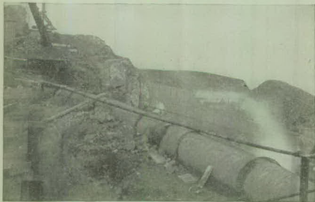
Cast Iron Pipe Exposed by Blasting
