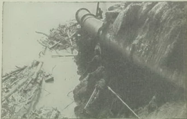
Pipe Line Completely Exposed by Washout of the Supporting Fill
