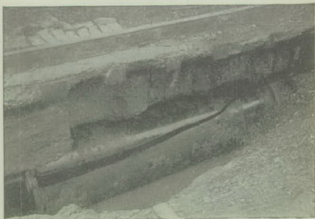
Pipe Broken Directly Under a Rail Joint
