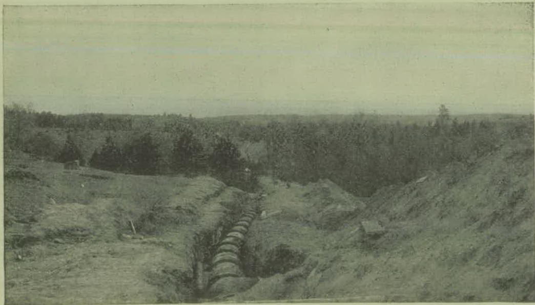
Large Cast Iron Pipe Through the Open Country
