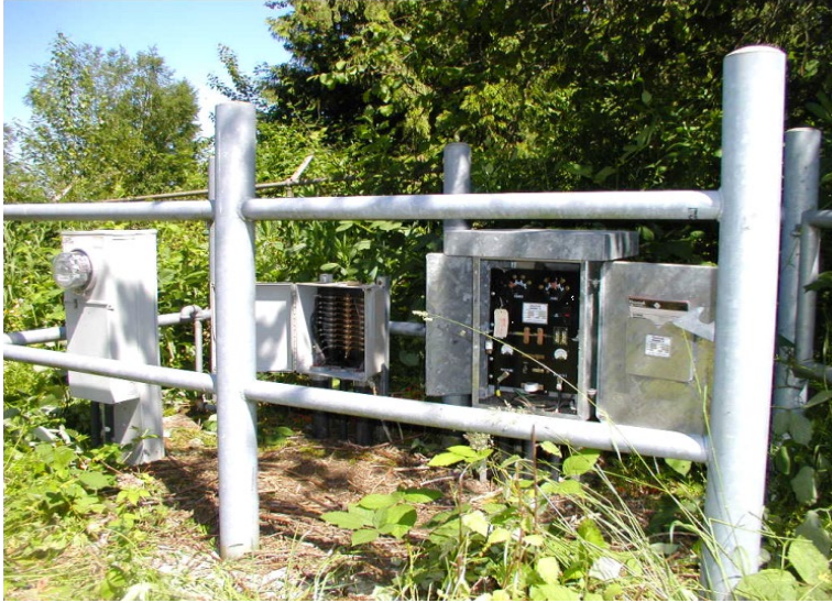
Figure 6-8 Typical Rectifier Installation
