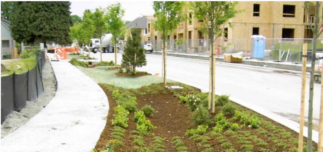
A newly planted natural drainage system.
