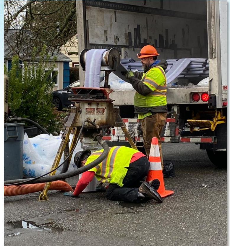
The photo is from SPU's recent Sewer Lining Contract, where Cured-in-Place Pipe (CIPP) lining is being installed.
