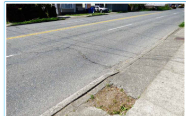
Damaged and narrow sidewalks along 23rd Ave S
