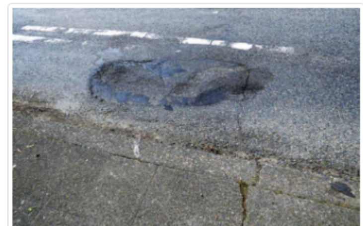
Potholes on 23rd Ave S
