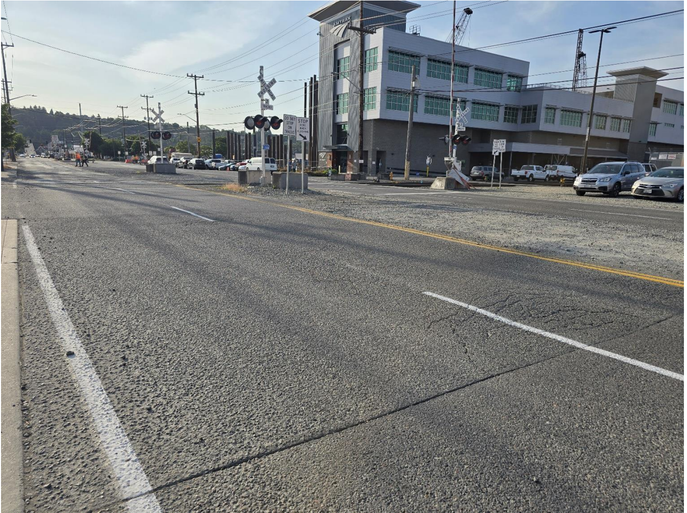
FIGURE 19- S HOLGATE ST AND DOT# 085583Y, ALLIGATORING, NW CORNER LOOKING SE
