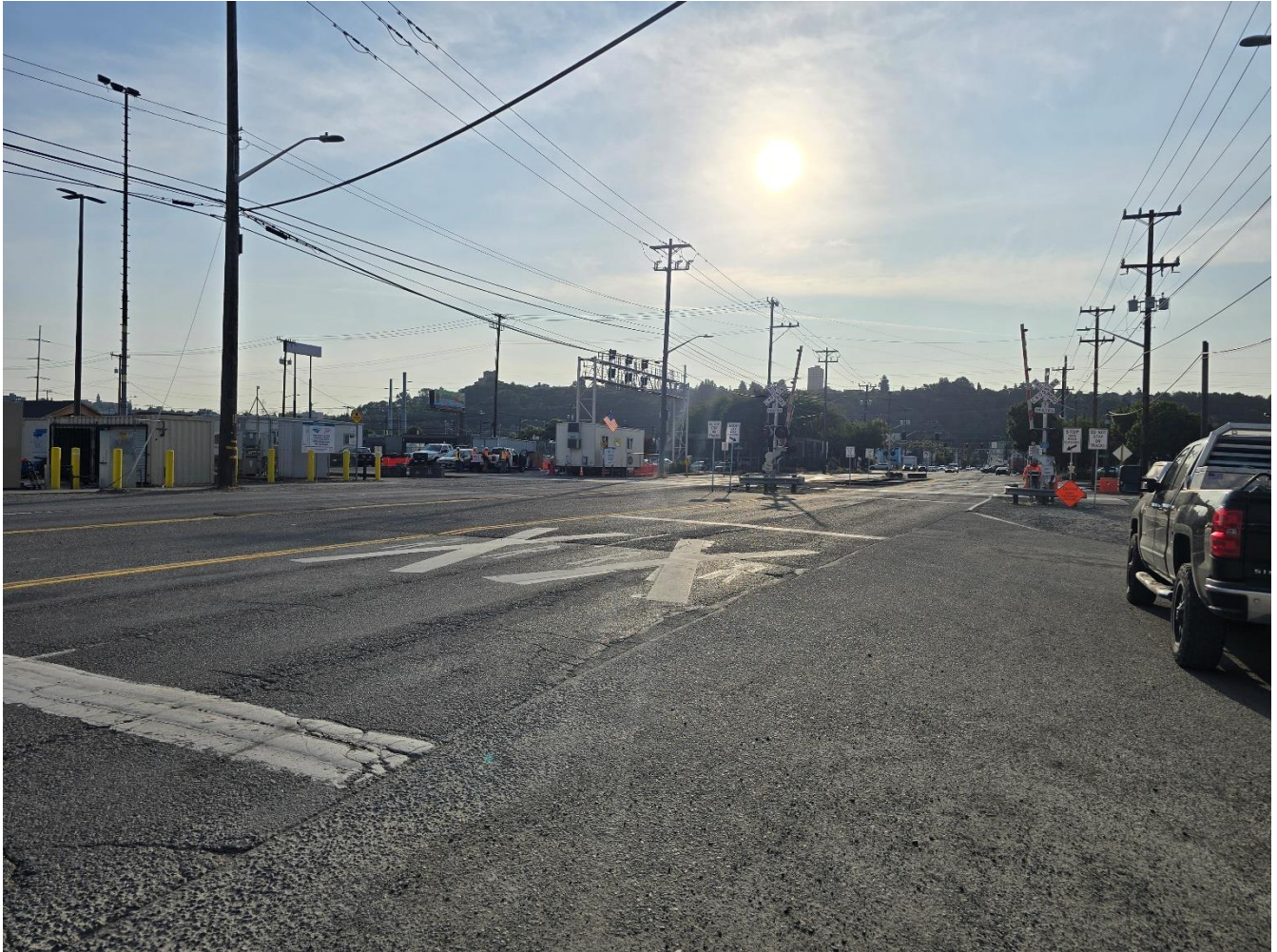
FIGURE 14-S HOLGATE ST AND DOT# 085583Y CROSSING, PAVEMENT CONDITION SHOWING ALLIGATORING OF PAVEMENT AND LATERAL CRACKING, SE CORNER LOOKING NE
