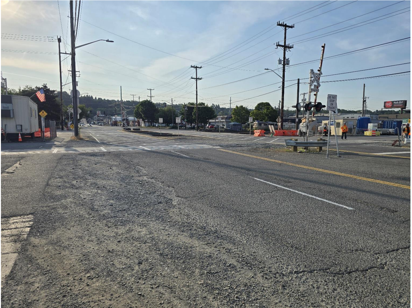
FIGURE 17-S HOLGATE ST AND DOT# 927461X, PAVEMENT CONDITION SHOWING ALLIGATORING, LONGITUDINAL AND LATERAL CRACKING, NW CORNER LOOKING SE
