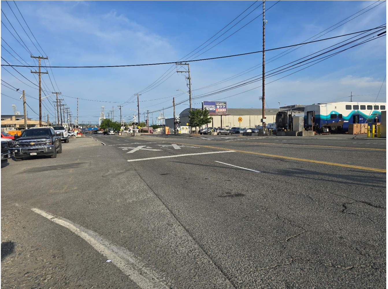
FIGURE 11-S HOLGATE ST AND DOT# 085583Y CROSSING, PAVEMENT CONDITION SHOWING ALIGATORING AND CRACKING, SW CORNER LOOKING NW
