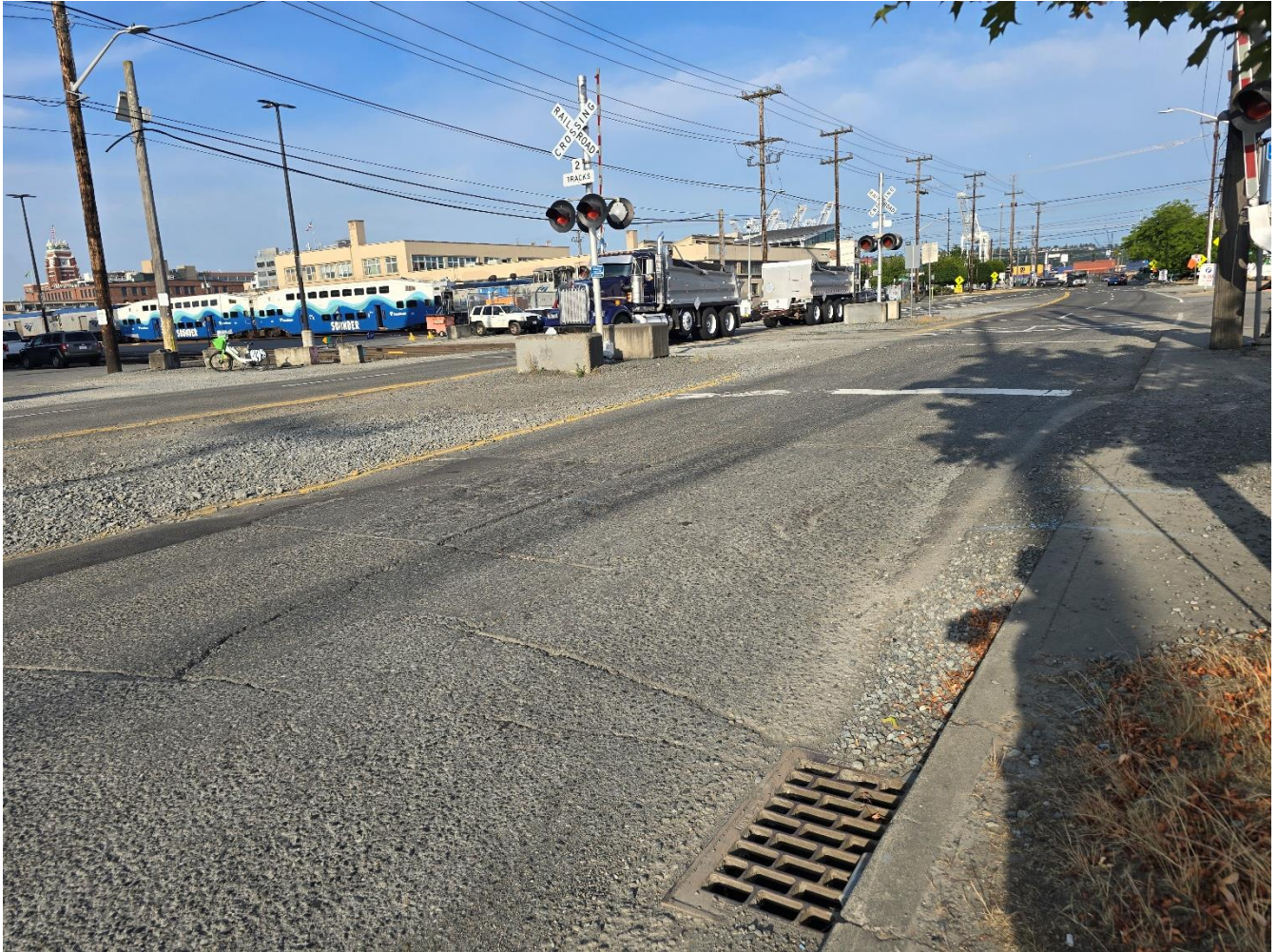
FIGURE 18-S HOLGATE ST AND DOT# 085583Y, ALLIGATORING, LONGITUDINAL AND LATERAL CRACKING, NE CORNER LOOKING SW
