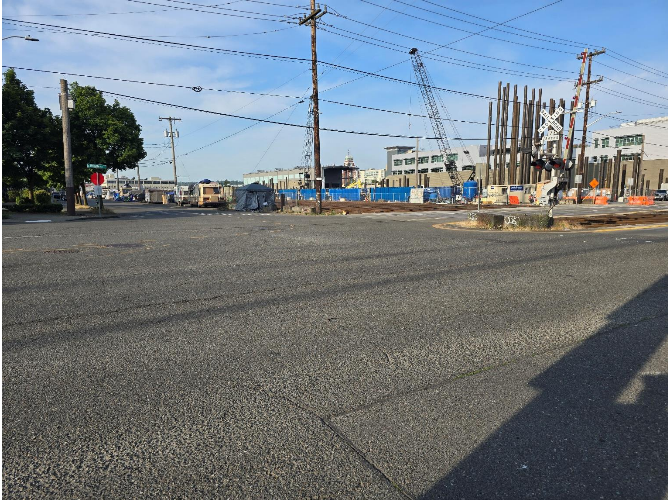
FIGURE 15-S HOLGATE ST AND 3 RD AVE S, NEAR DOT# 927461X, PAVEMENT CONDITION SHOWING LONGITUDINAL CRACKING AND PATCHING, NE CORNER LOOKING SW
