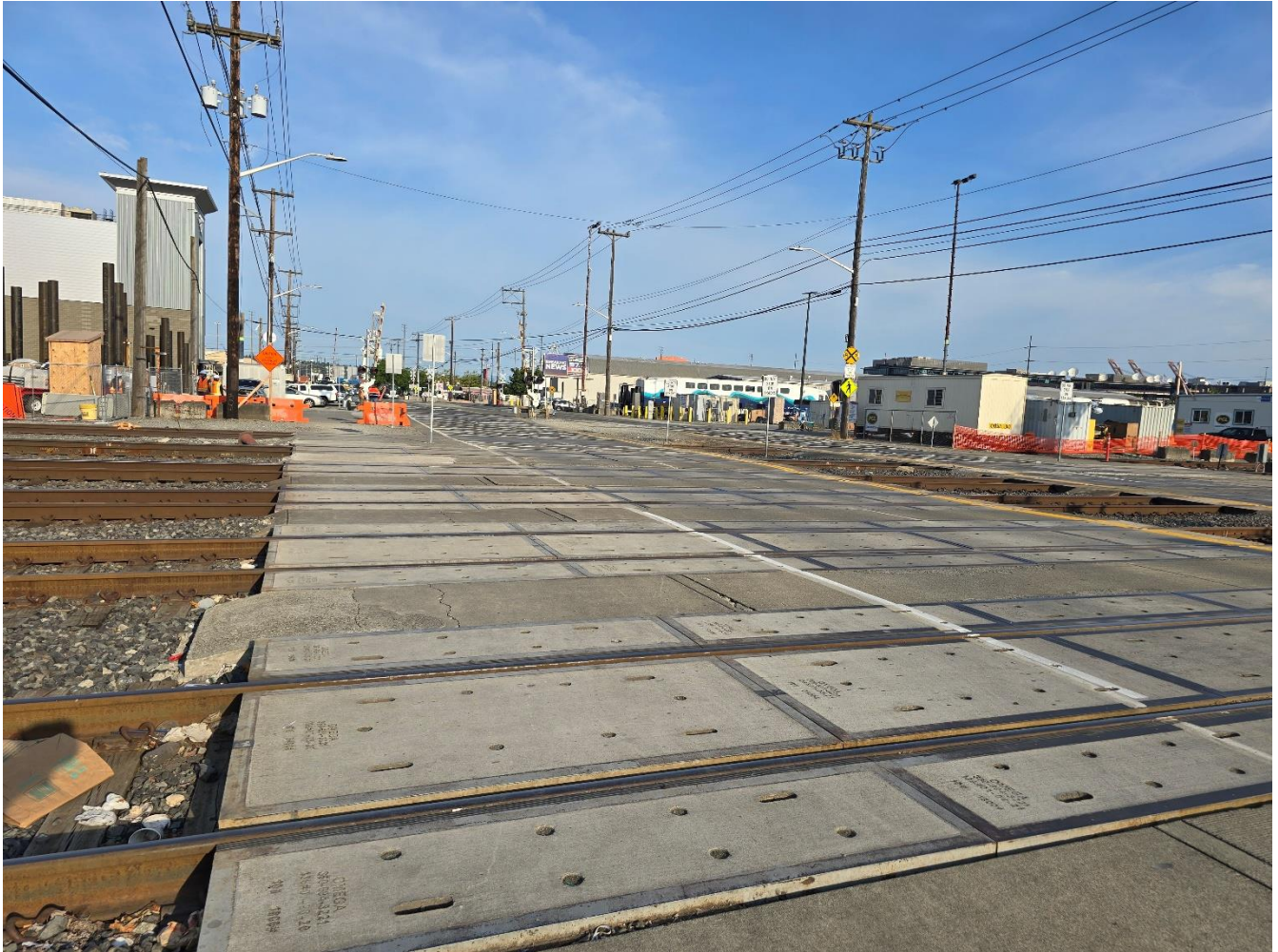
FIGURE 13-S HOLGATE ST AND DOT# 927461X CROSSING, PAVEMENT CONDITION SHOWING FAILURE OF PAVEMENT BETWEEN RAIL CROSSING, SE CORNER LOOKING NW
