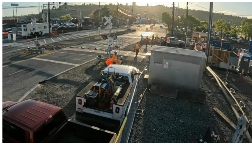
FIGURE 42: VIDEO CAPTURE OF AMTRAK WORKERS WALKING ACROSS THE TRACKS WHILE GATES ARE DOWN (APRIL 22, 2025)
