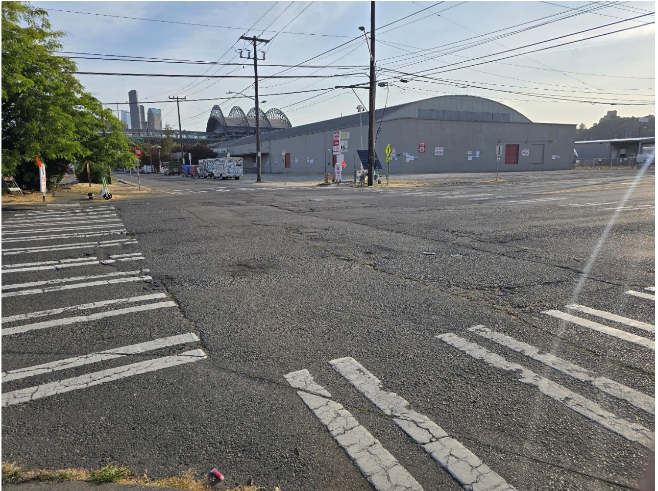
FIGURE 10-S HOLGATE ST AND OCCIDENTAL AVE S, PAVEMENT CONDITION SHOWING ALIGATORING AND CRACKING, SW CORNER LOOKING NE
