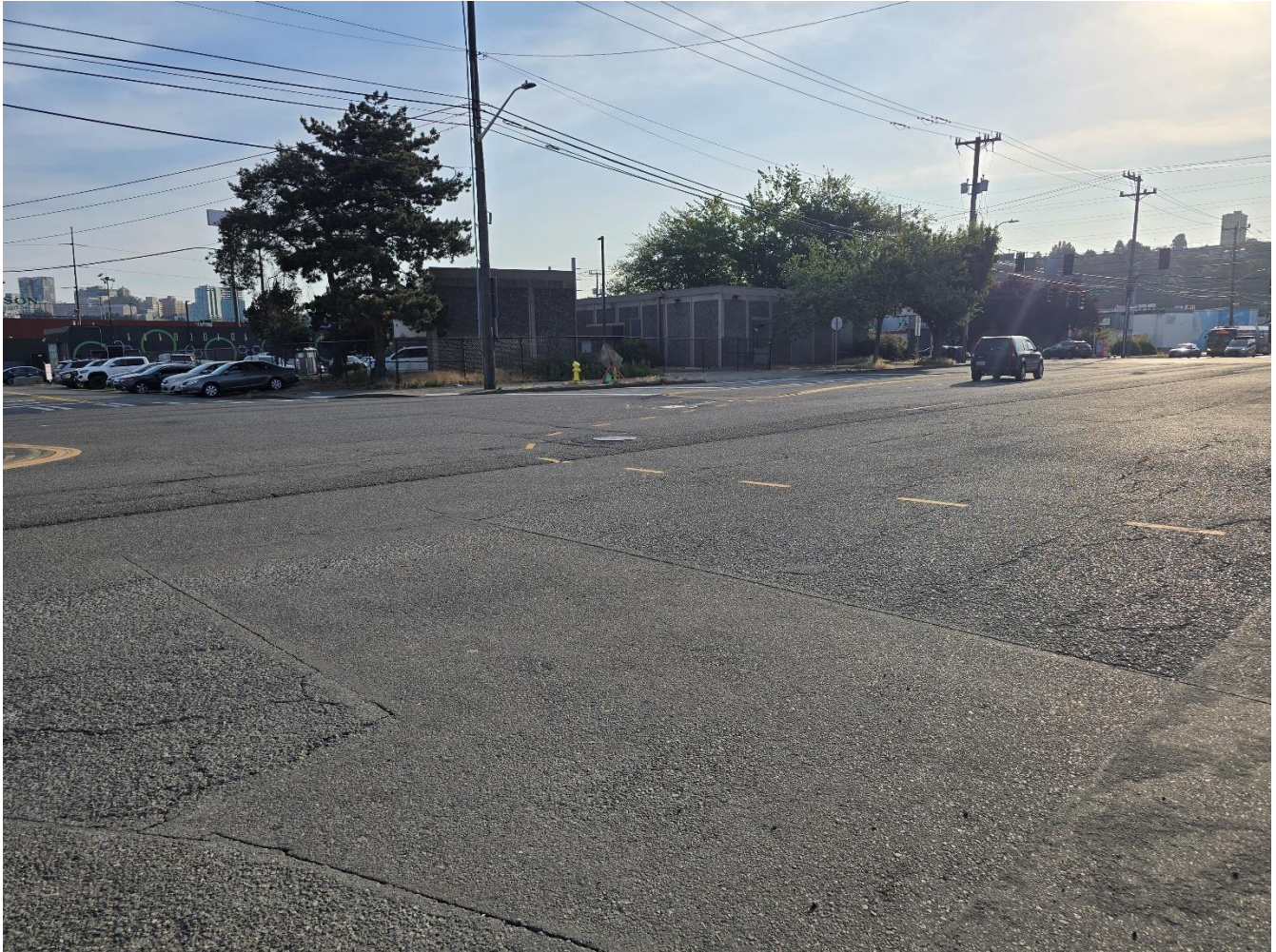
FIGURE 16-S HOLGATE ST AND 3RD AVE S, PAVEMENT CONDITION SHOWING ALLIGATOR CRACKING AND PATCHING, SW CORNER LOOKING NE
