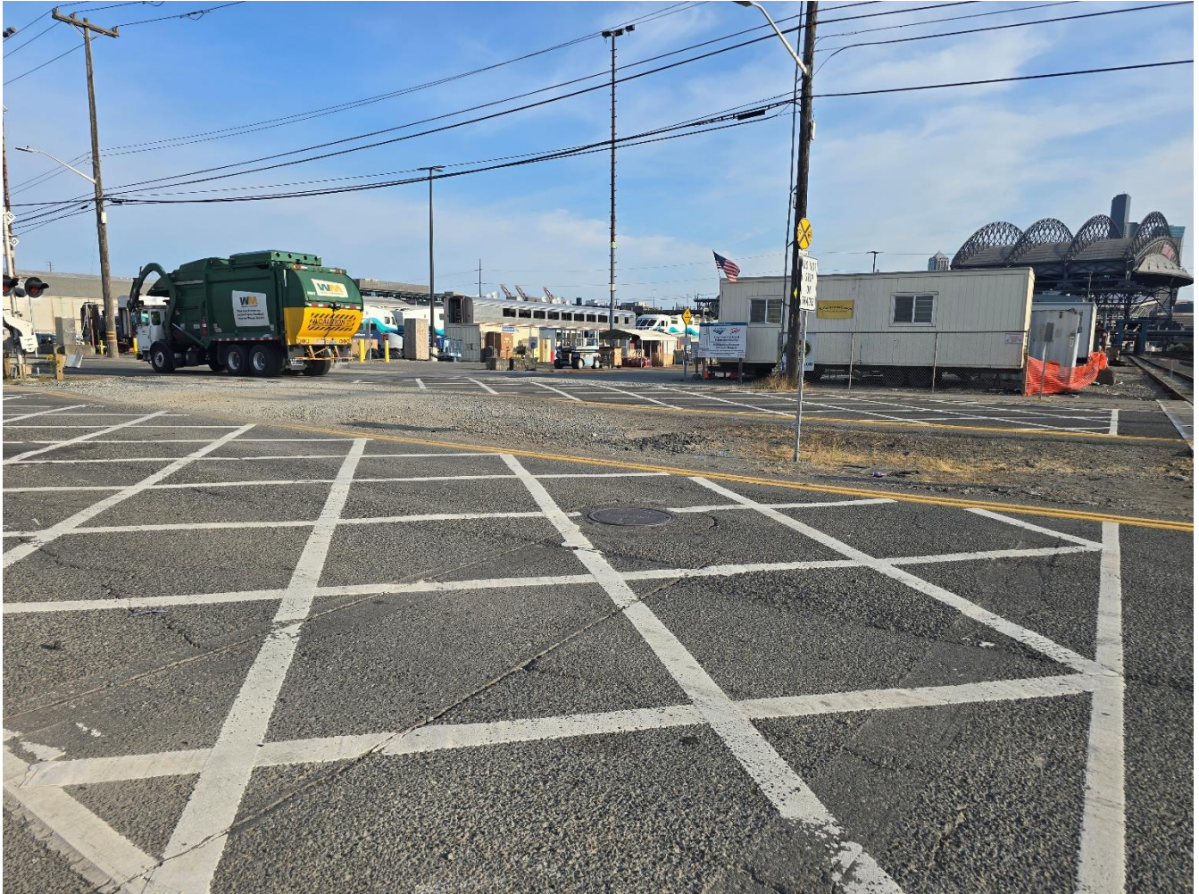
FIGURE 12-S HOLGATE ST BETWEEN DOT# 085583Y AND 927461X CROSSING, PAVEMENT CONDITION SHOWING ALIGATORING AND TRENCH REPAIR, SW CORNER LOOKING NW
