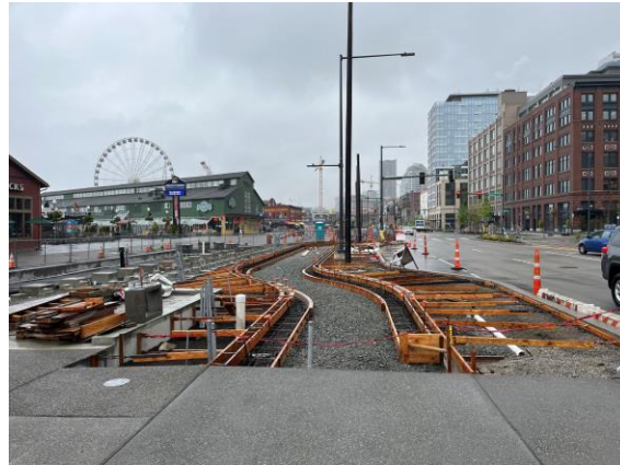
Waterfront bike path under construction between Yesler Way and Virginia St, planned opening by 2024
