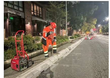
SDOT crews installing new better bike lane barriers on E Yesler Way.
