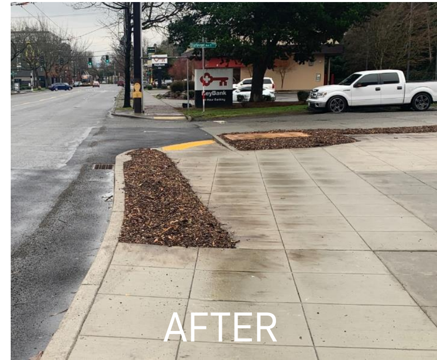
Before and after new extended curb at Rainier Ave S and S Sturtevant St.
