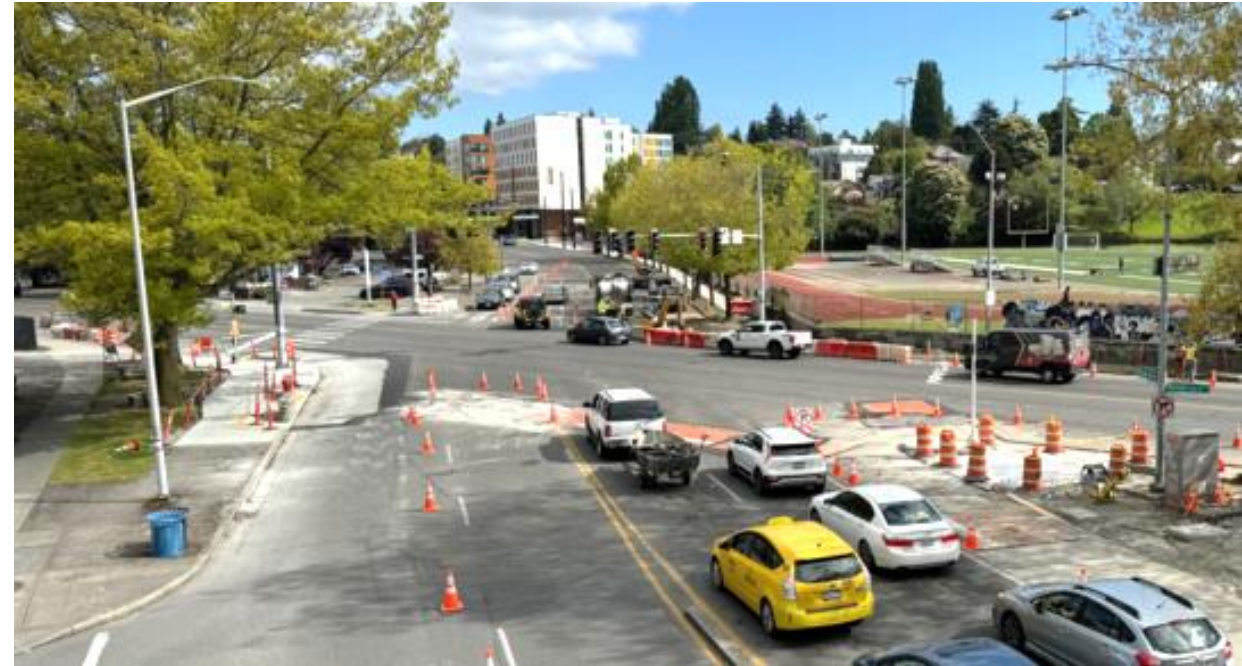
Construction underway at the MLK Jr Way S and Rainier Ave S intersection as part of MLK Jr Way Safety Project
