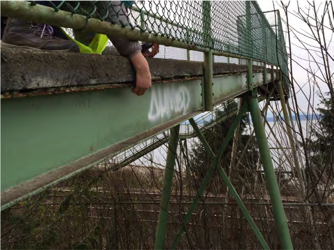
Figure 9 Corrosion at Steel Beam Top Flange
