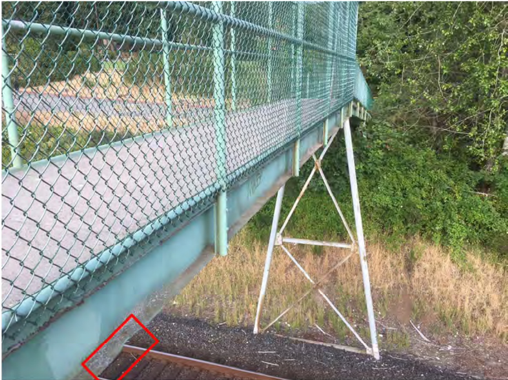
Figure 3 Bridge Steel Beam Bottom Flange Dent
