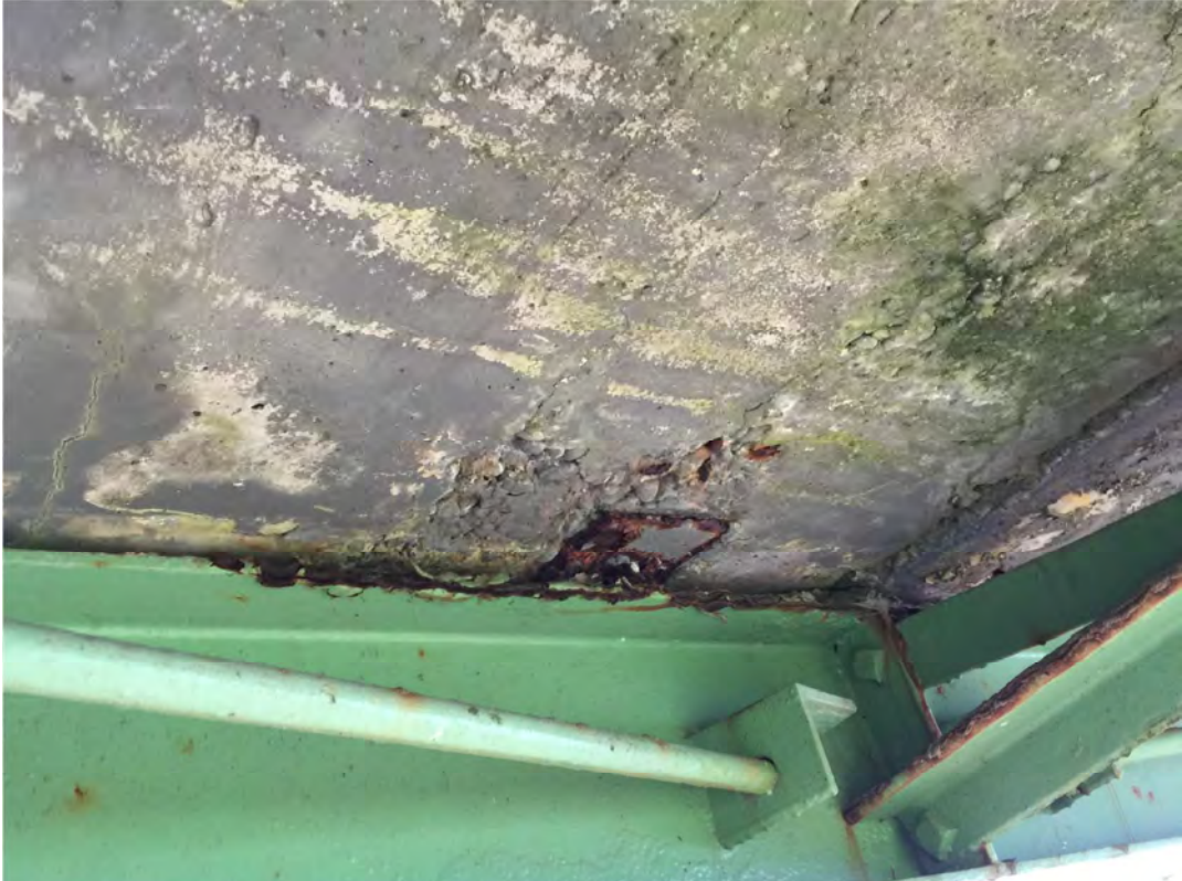
Figure 5 Corrosion and Spalling at Bolt Connection with Precast Slab
