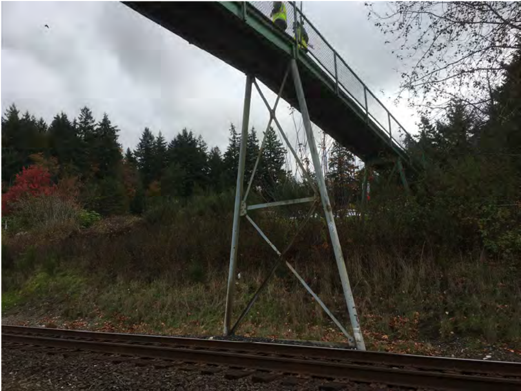
Figure 6 Pier with Corrosion Members at the Other Side of BNSF Tracks
