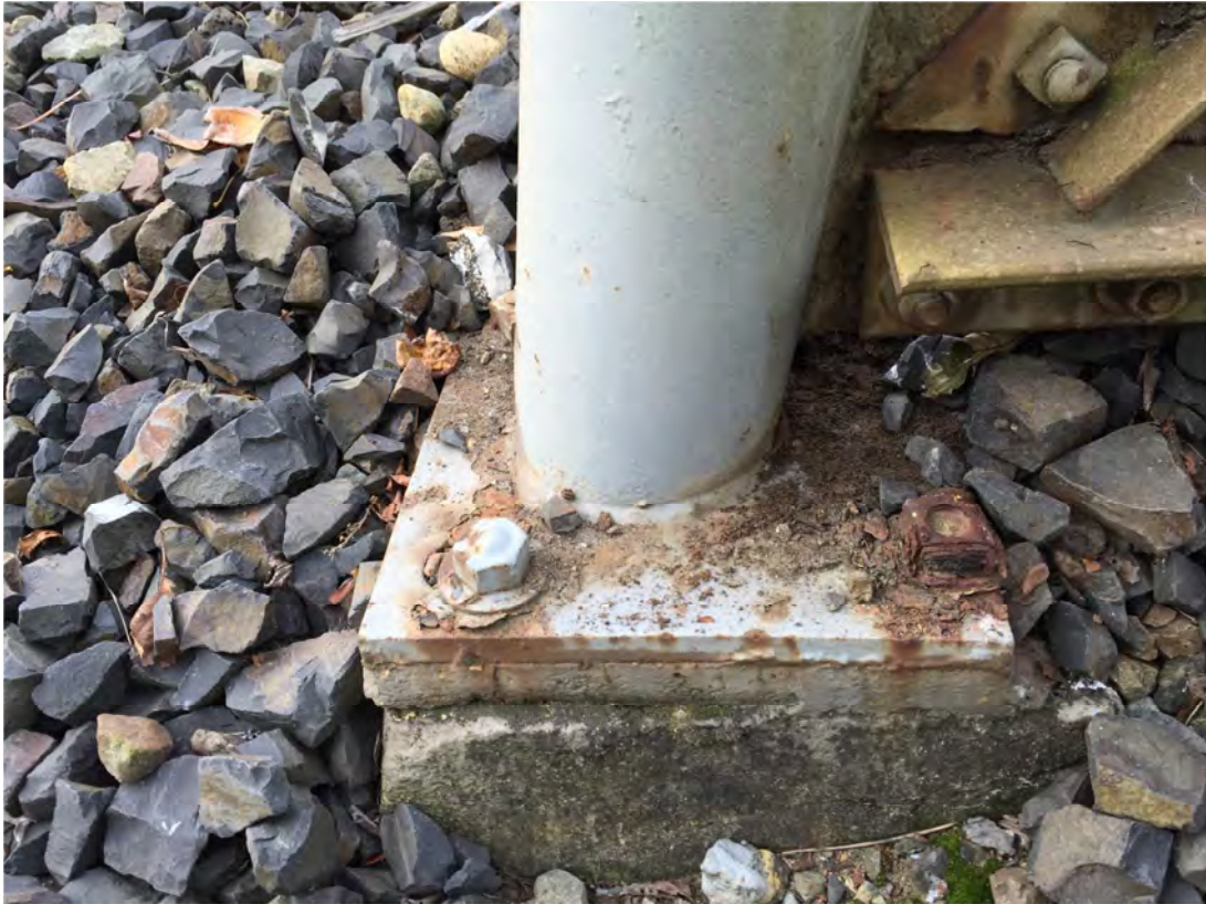
Figure 7 Corrosion at Pier Pipe Base Plate Anchor
