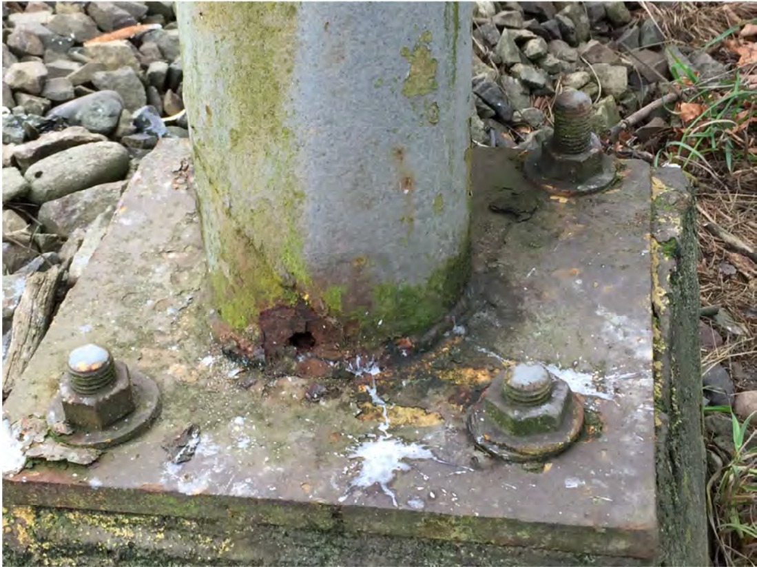
Figure 8 Corrosion at Pier Pipe Base with Visible hole
