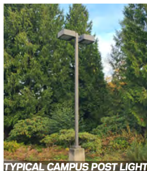
TYPICAL CAMPUS POST LIGHT
