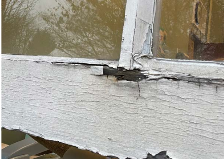
Dry rot at intersection of muntins and sash
