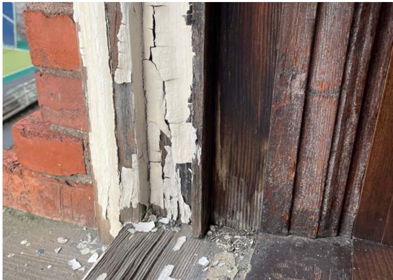
Exterior paint failure resulting in weathered bare wood at frame and sill
