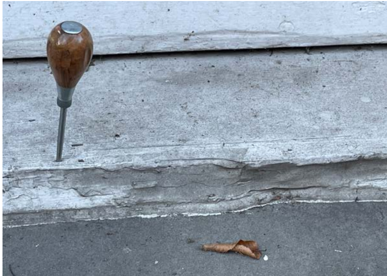
Advanced wood rot at sills
