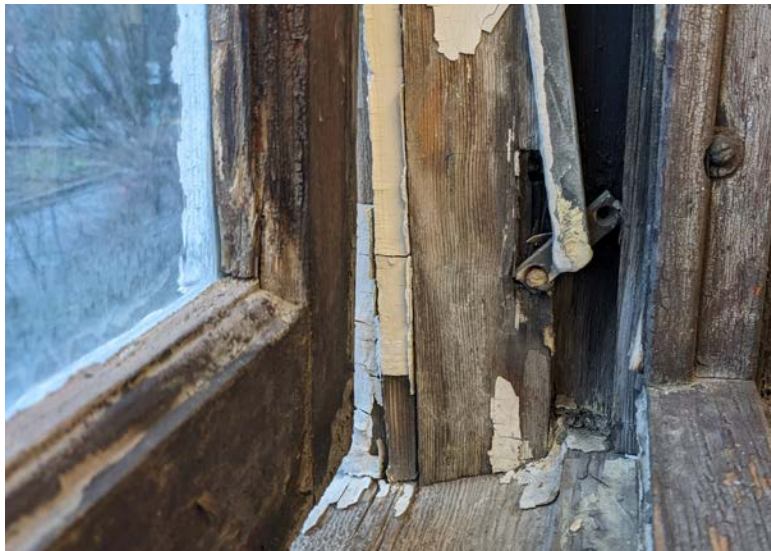
1916 tilt hardware in very bad condition
