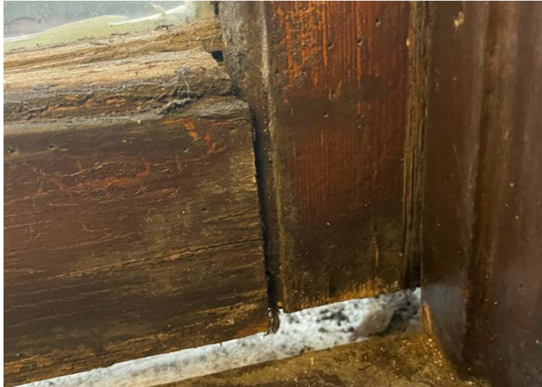
Separation between stile and bottom rail
