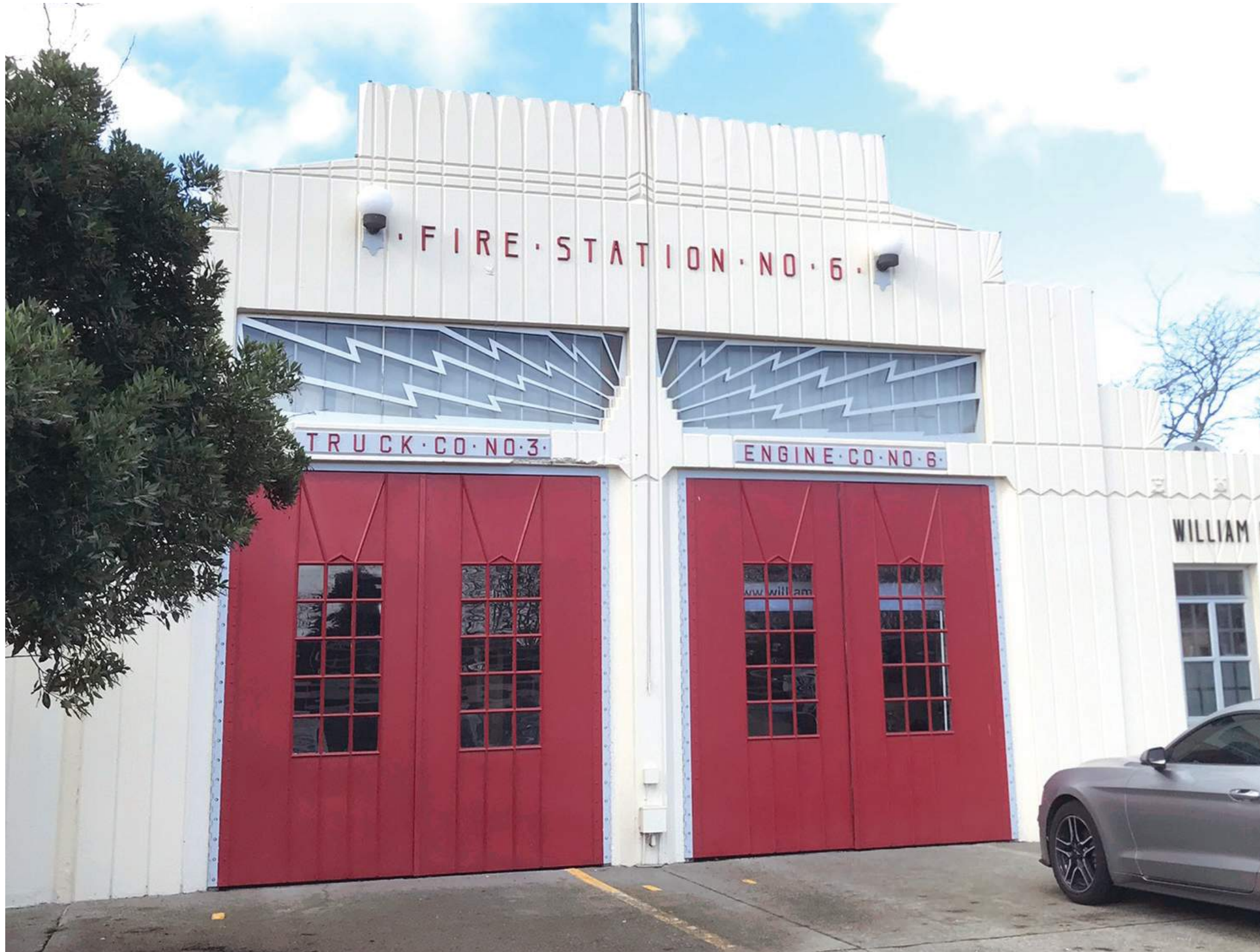
figure 52: Current condition of apparatus bay doors, 1986 replica of original
