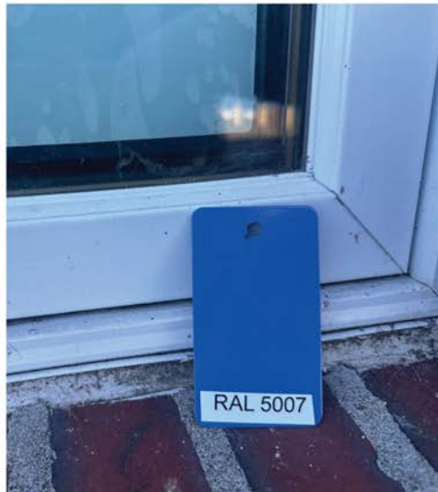
in proximity to other materials on building
