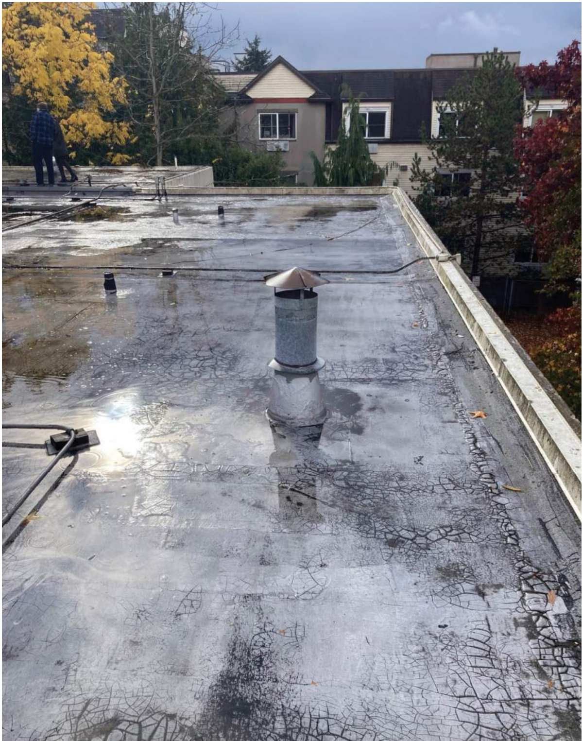
figure 8: Ponding on current roof from insufficient slope. Existing flashing detail preserves appearance of parapet.
