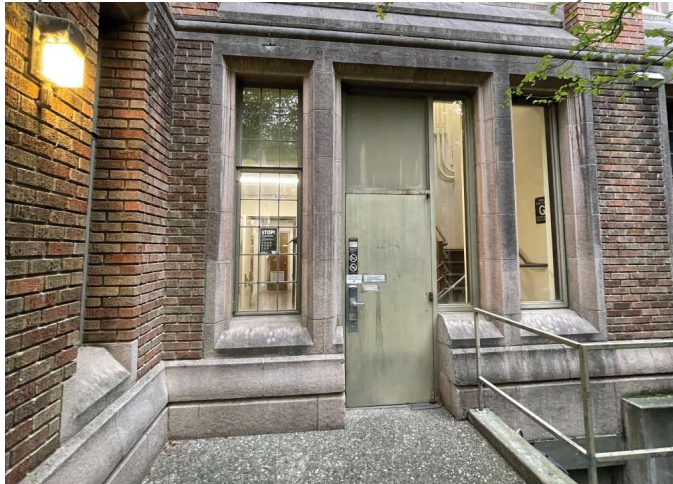
Southwest entry added in 1971 after removal of the central entry doors and arcade.
