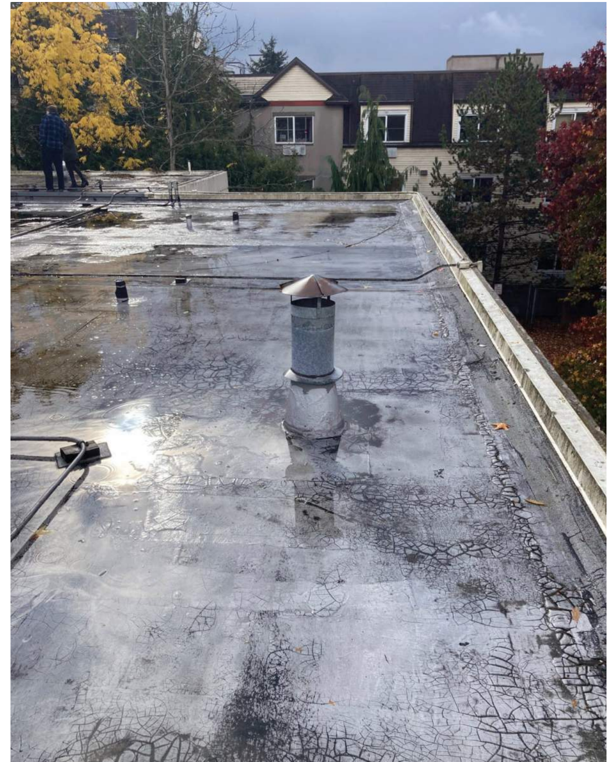
figure 7: Ponding on current roof from insufficient slope. Existing flashing detail preserves appearance of parapet.
