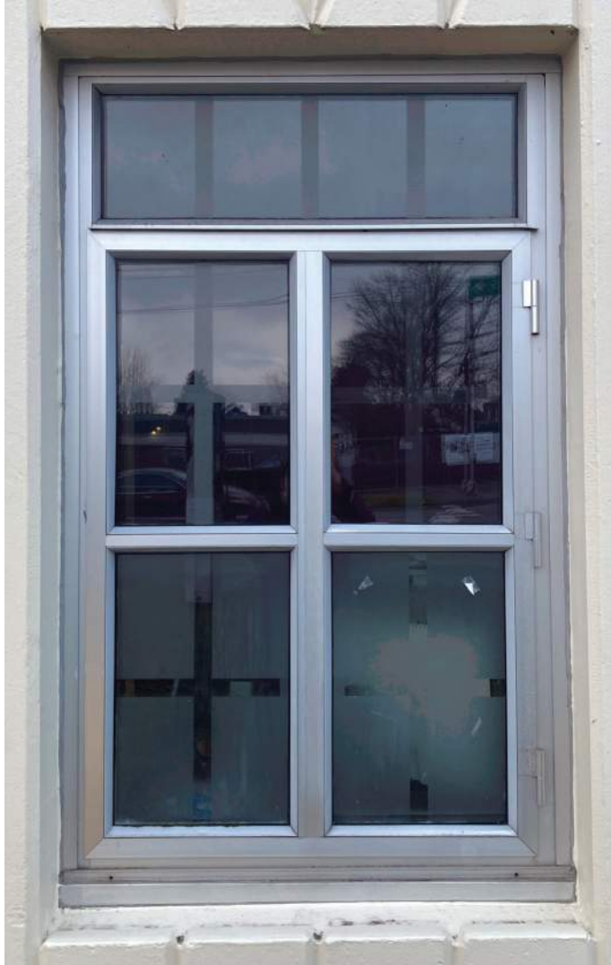
figure 12: Existing 1999 aluminum window with etched "panes."
