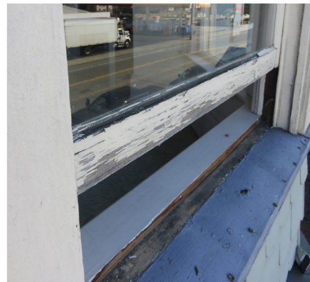
MISSING PUTTY, DAMAGE SILL COVER
