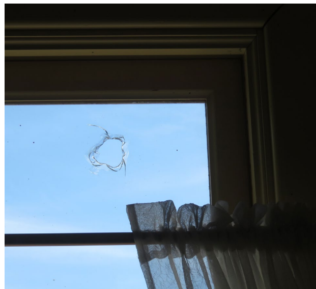
HOLE IN GLAZING
