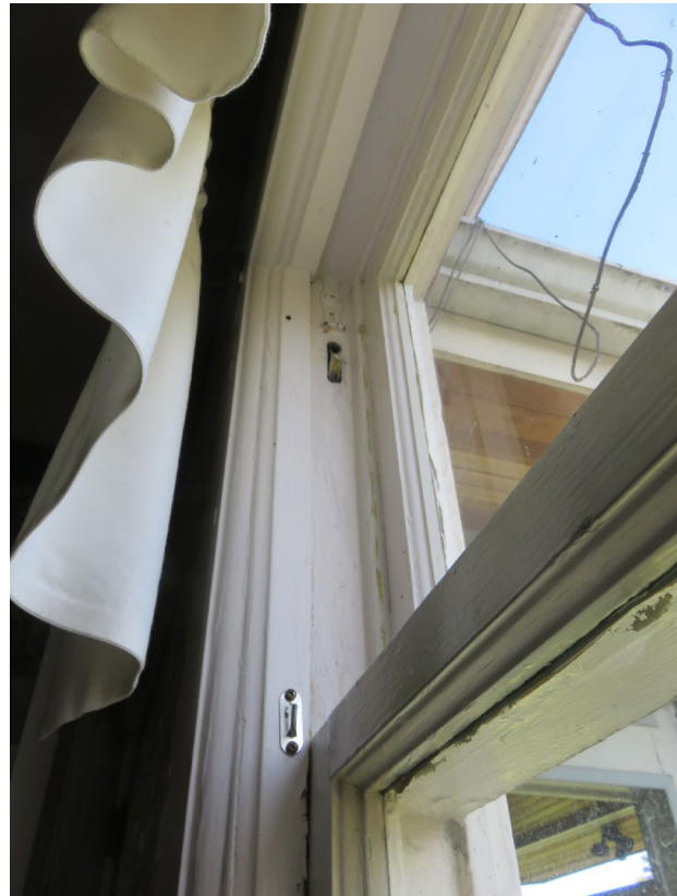
MISSING ROPES & WEIGHTS
