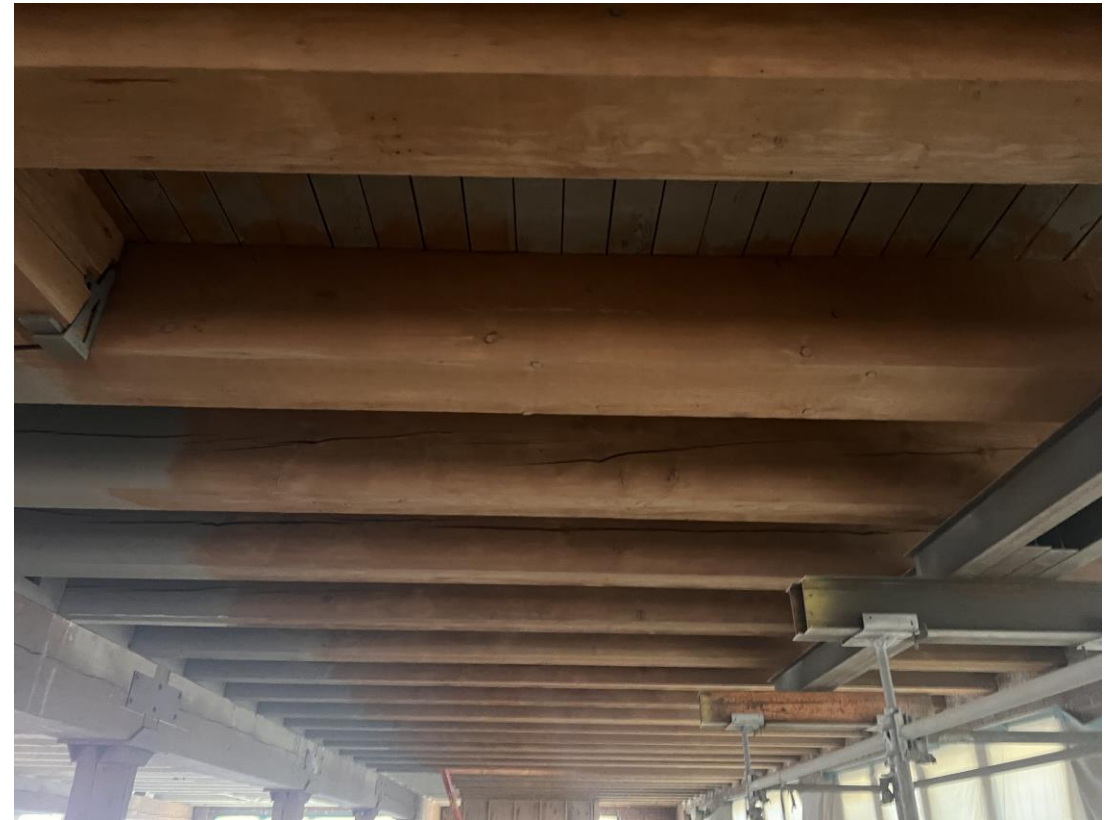
8/2/2023 – Exposed Beams with No Ductwork
