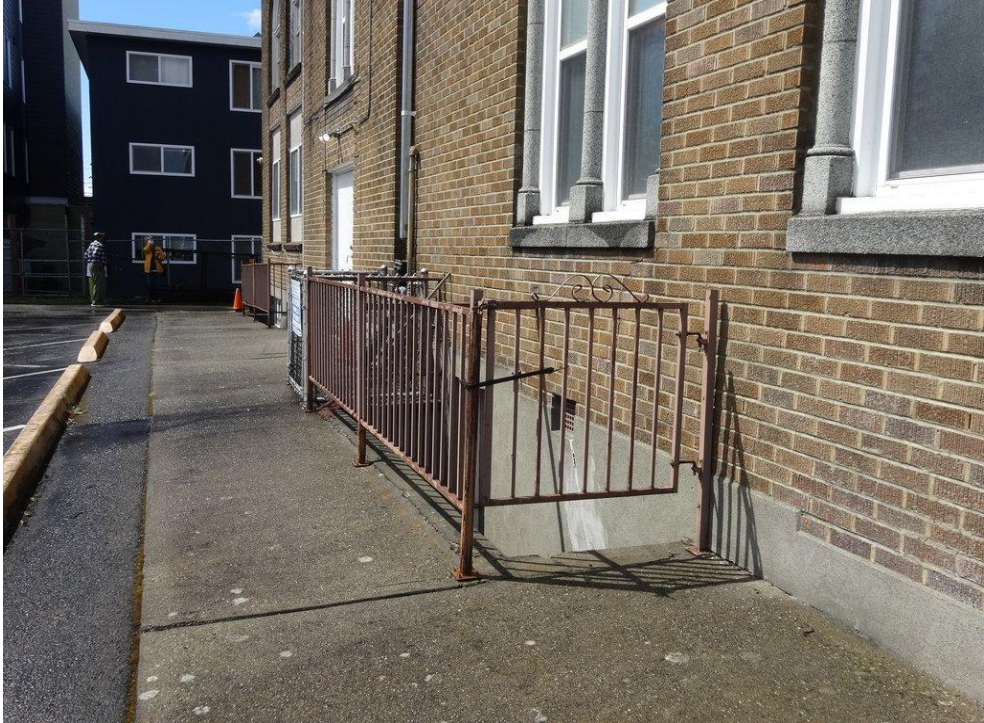
B18. Limited-access entrance to basement. Photo taken from parking lot, facing west. May 7, 2021.
