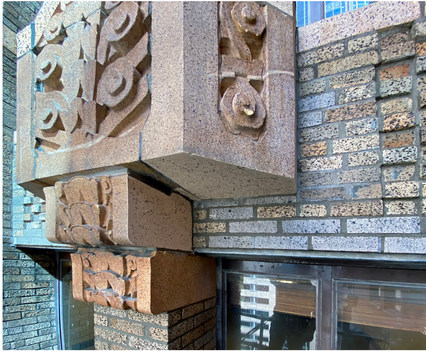
DETAIL OF LINTEL WITH TERRACOTTA ACCENT PIECE REMOVED AND PATCHED WITH BRICK TO MATCH EXISTING SURROUNDING FIELD BRICK.
