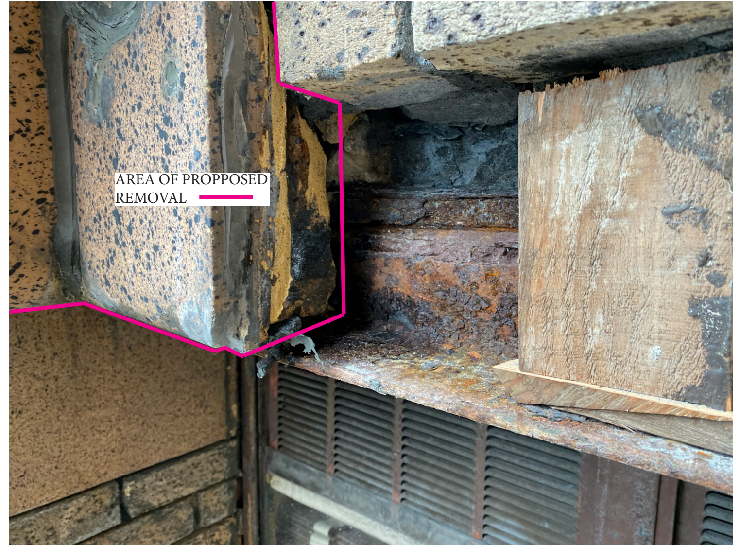
DETAIL OF DAMAGE AT LINTEL, BRICK, AND TERRACOTTA MEDALLION INTERFACE, TYPICAL OF ALL LOCATIONS TO VARYING DEGREES.
