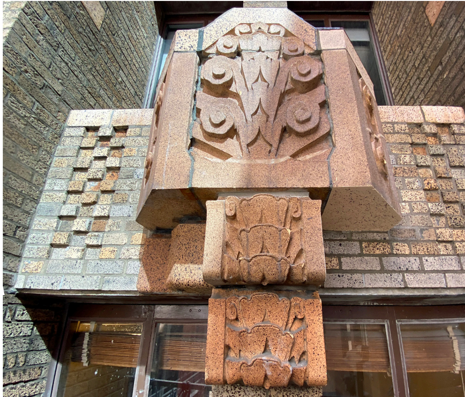
DETAIL OF LINTEL WITH TERRACOTTA ACCENT PIECE REMOVED AND PATCHED WITH BRICK TO MATCH EXISTING SURROUNDING FIELD BRICK. LEFT SIDE SHOWS ORIGINAL ACCENT PIECE FOR COMPARISON.
