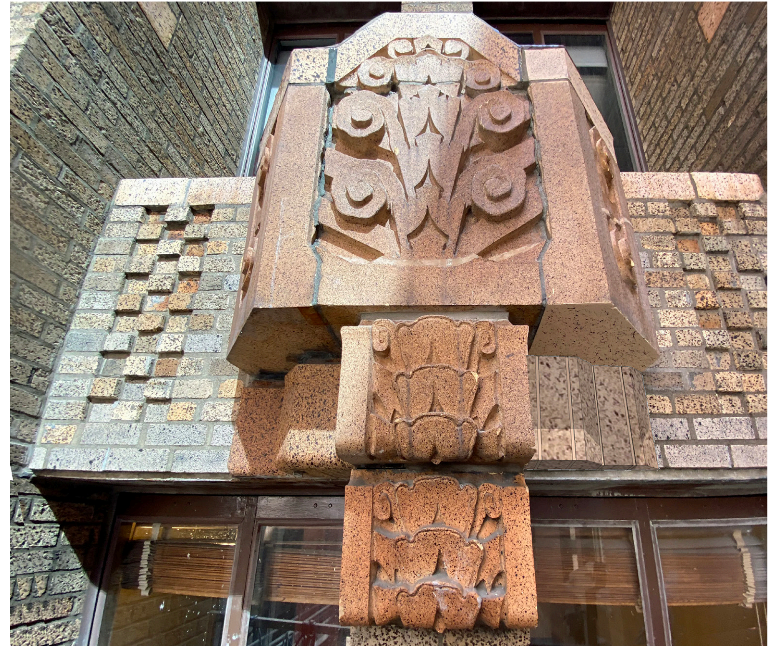
DETAIL OF LINTEL WITH TERRACOTTA ACCENT PIECE REMOVED AND REPLACED WITH COLOR MATCHED BRICK TO MIMIC EXISTING SUPPORT SHAPE. THE GROUT WOULD BE COLOR MATCHED TO BRICK TO MAKE THE ACCENT BRICK APPEAR AS MONOLITHIC AS POSSIBLE. THE LEFT SIDE SHOWS ORIGINAL ACCENT PIECE FOR COMPARISON.
