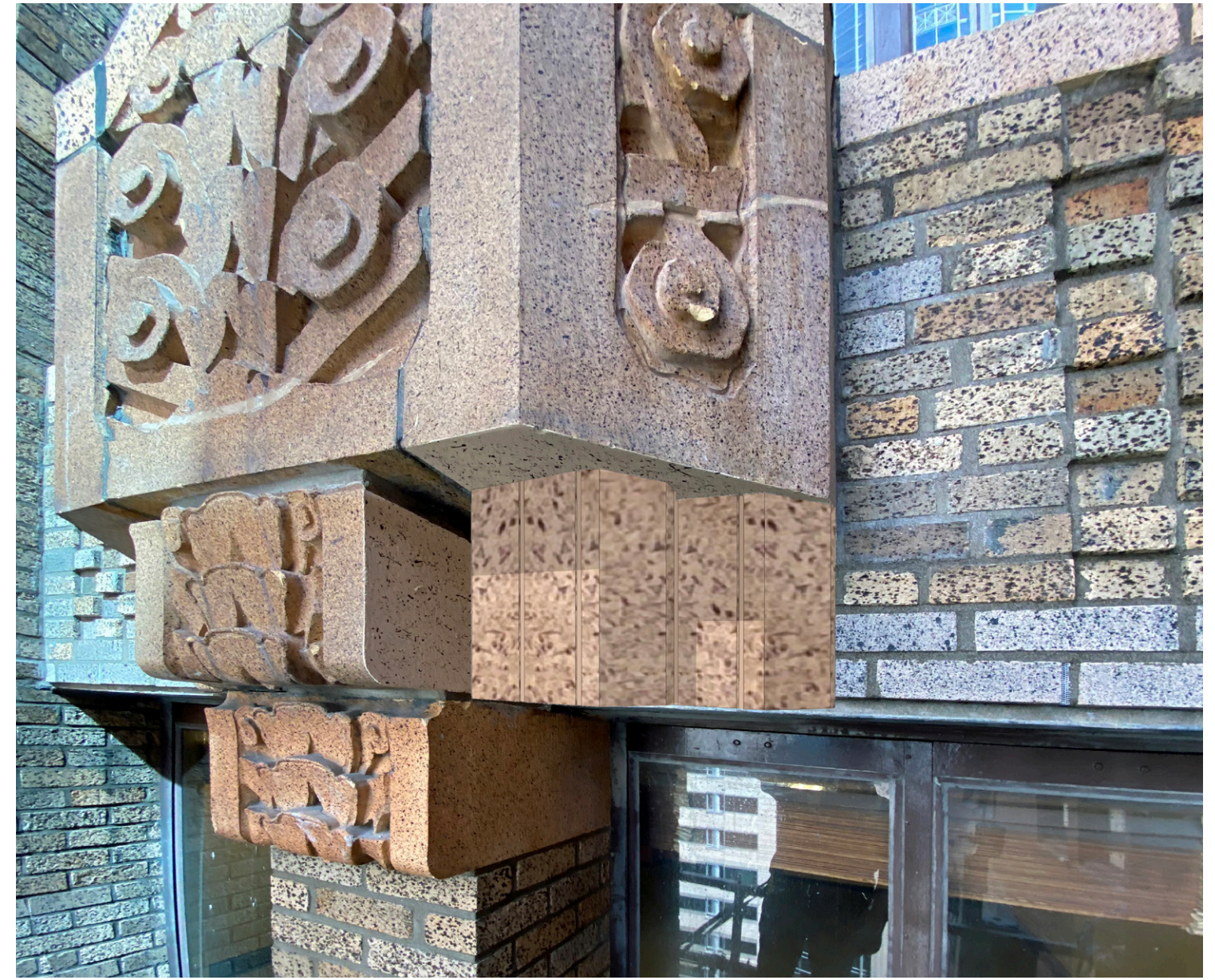
DETAIL OF LINTEL WITH TERRACOTTA ACCENT PIECE REMOVED AND REPLACED WITH COLOR MATCHED BRICK TO MIMIC EXISTING SUPPORT SHAPE. THE GROUT WOULD BE COLOR MATCHED TO BRICK TO MAKE THE ACCENT BRICK APPEAR AS MONOLITHIC AS POSSIBLE. THE LEFT SIDE SHOWS ORIGINAL ACCENT PIECE FOR COMPARISON.
