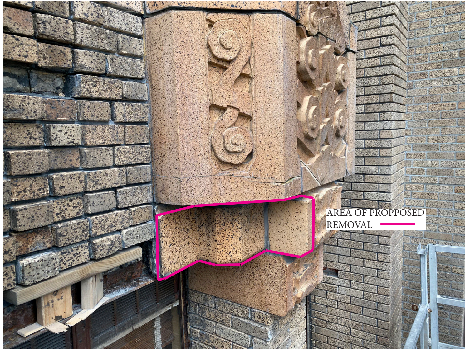
DETAIL OF DAMAGE AT LINTEL, BRICK, AND TERRACOTTA MEDALLION INTERFACE, TYPICAL OF ALL LOCATIONS TO VARYING DEGREES.
