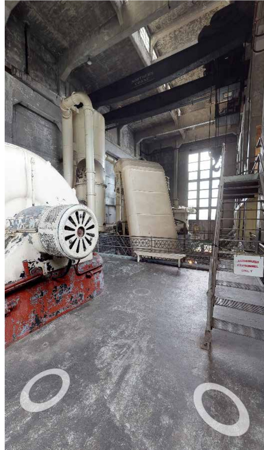
The Engine Mezzanine
