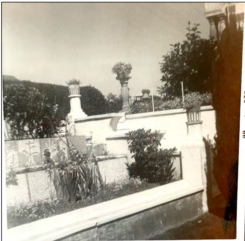
Fig. 82 – 1966 photo of the retaining wall and steps at the southwest corner of the house. Note pebble mosaic concrete tiles forming garden bed terraces, which remain intact, as do the steps. (Retaining wall with integral bench no longer intact). (VC)
