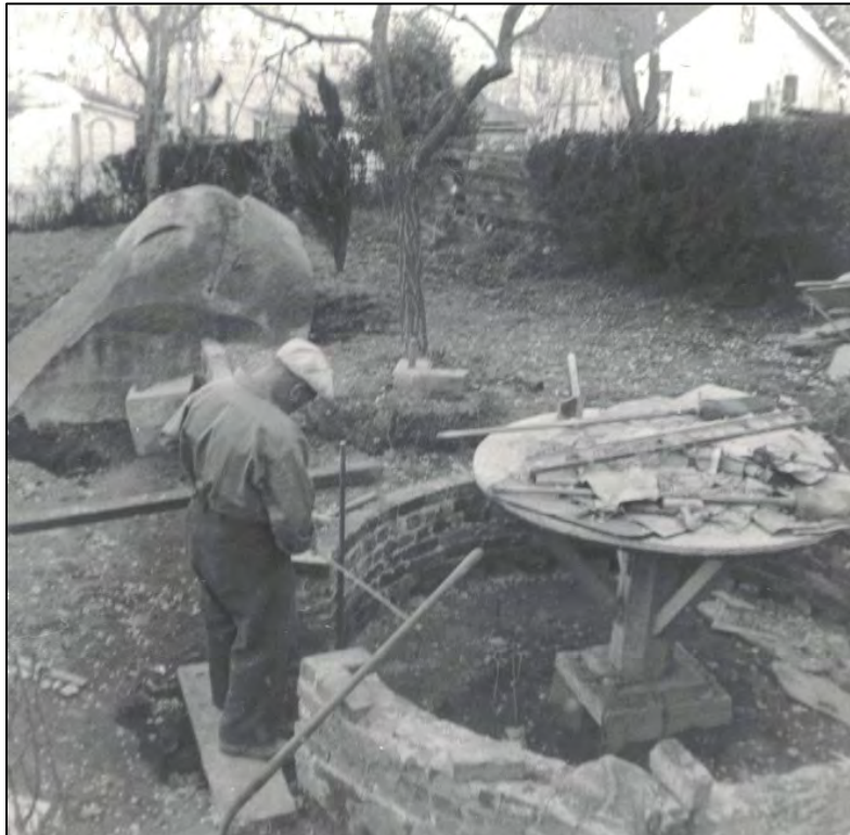
Fig. 87 – 1940s view of Fausto building a retaining wall and one of the terrazzo tables. The glacial erratic boulder on the property is visible at left. (No longer extant). (VC)
