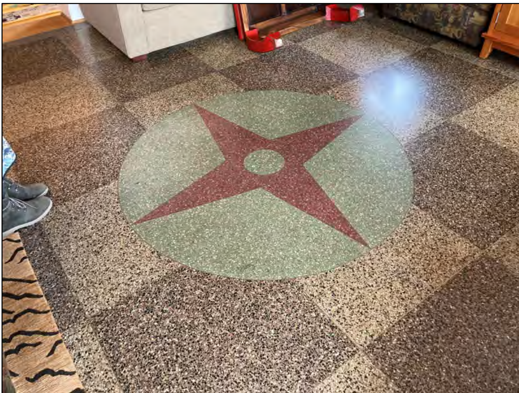
Fig. 48 – Interior, basement level, showing present living room at northeast building corner, and original terrazzo floors. The Cettolins used this room as the dining room.
