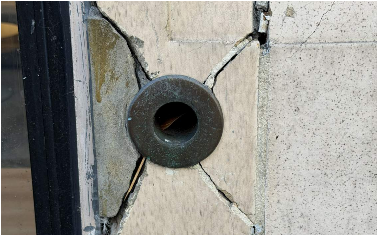
THE DOYLE BUILDING - FACADE DETAIL (PREVIOUS REPAIRS AT OVERFLOW DRAIN)
