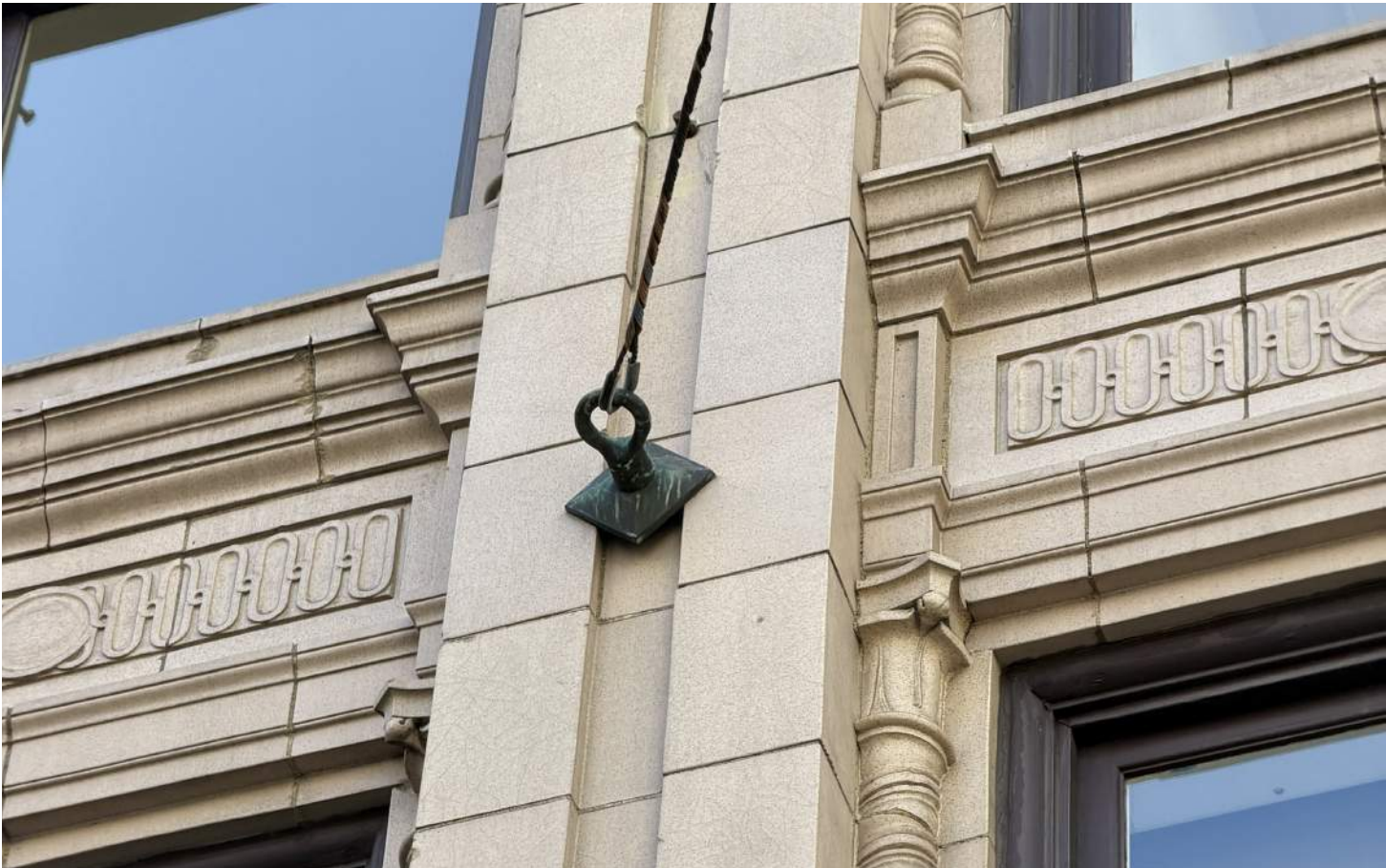
THE DOYLE BUILDING - FACADE DETAIL (OVERHEAD CABLE ATTACHMENT)
