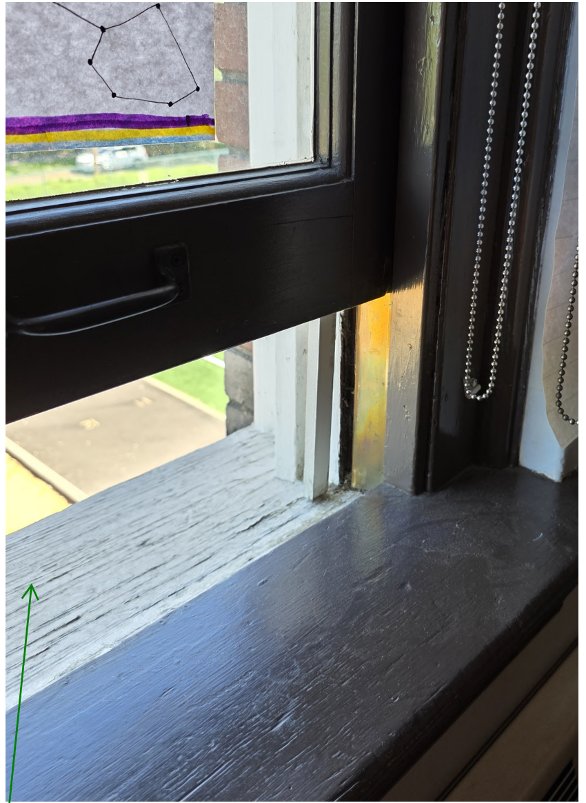
moderate weathering on exterior window sill.
