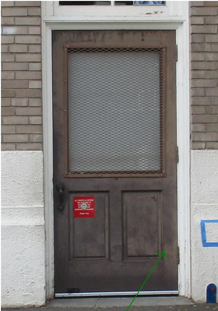
Exterior paint is faded
