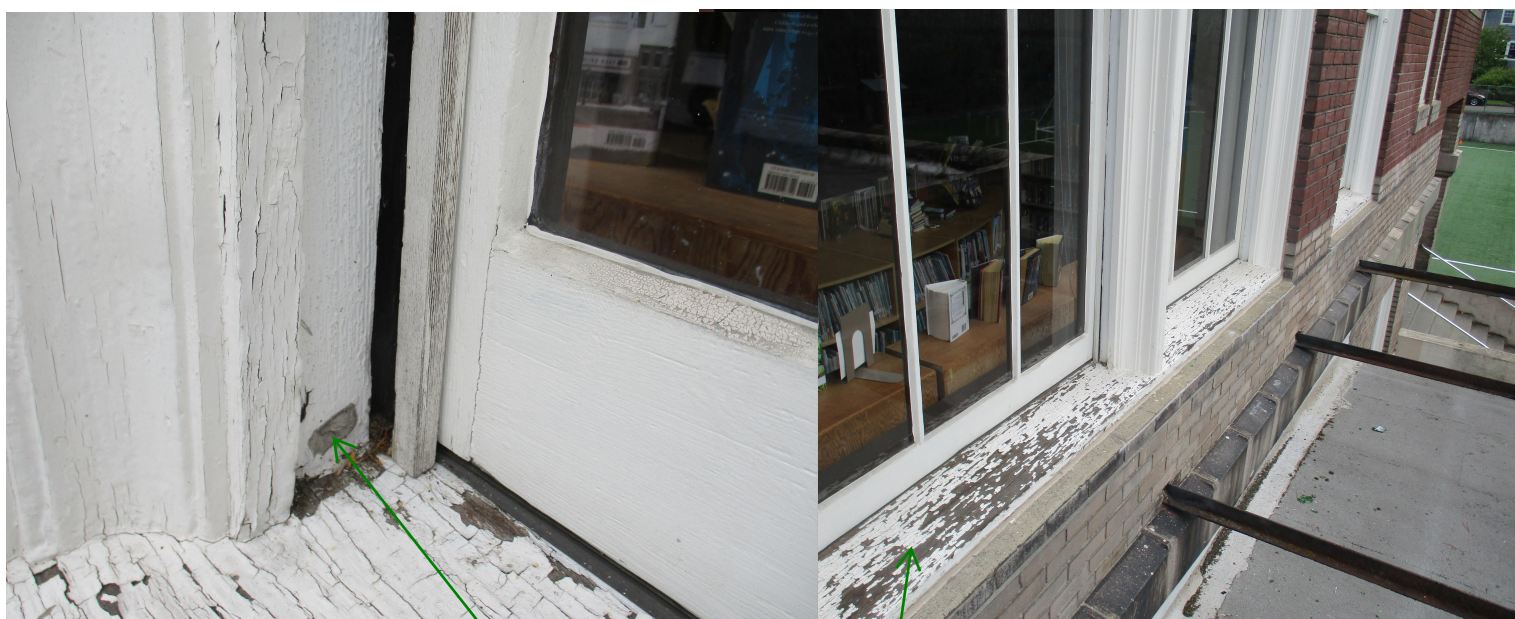
Faded paint on the exterior window sills
