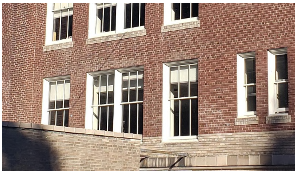
The Second floor Library window are in fair condition with minor chips in the paint observed on the jambs and some damage observed on the exterior sill due to its skyward facing nature.
