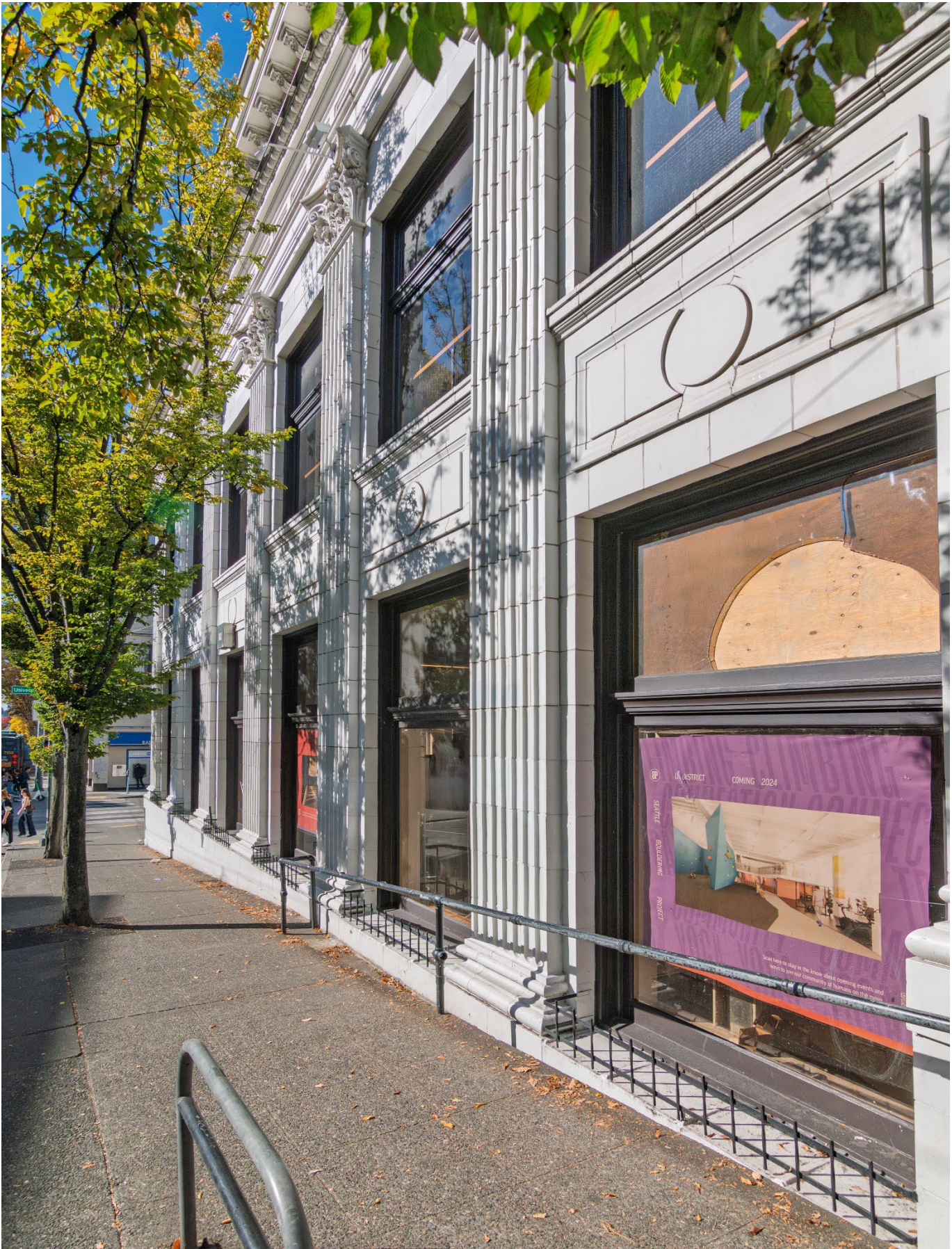
During final LL construction- Fixing broken glass at LL phase. Façade looking NW.
