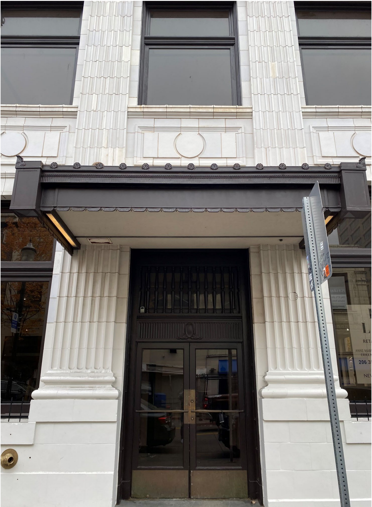
During LL construction- Rehab canopy / front doors, etc. - post LL work. Looking E.
