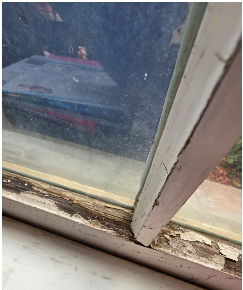
Classroom 2 - South Elevation Paint failure and wood deterioration typical at Window Rails & Muntins.
