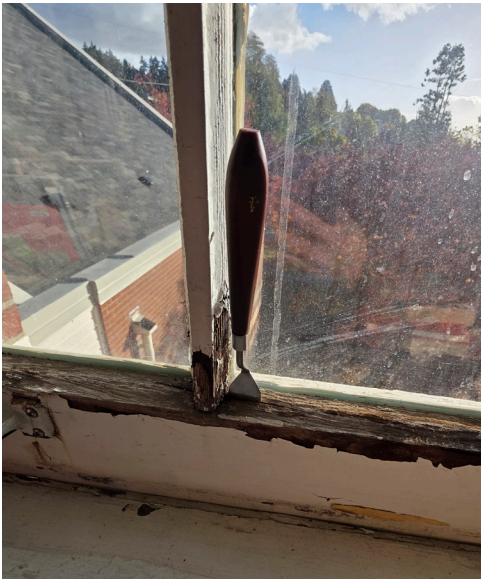
Classroom 17 - South Elevation Bottom Rail is completely Rotted
