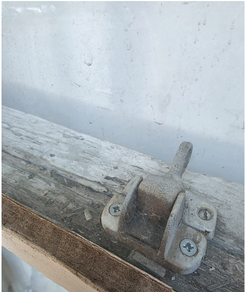
Classroom 1 - South Elevation Paint Failure and extensive wood Deterioration at upper sash bottom rail.
