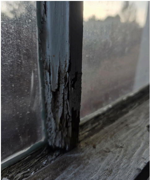
Classroom 19 - South Elevation Paint failure and wood deterioration at rail and muntin.
