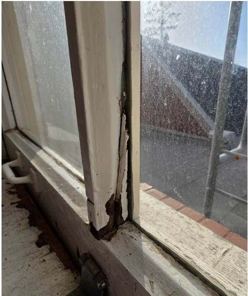
3rd Floor Hallway - West Elevation Middle operable sashes, base of muntin cracked.
