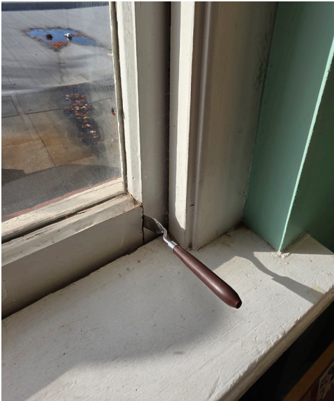
3rd Floor Hallway - West Elevation Damaged but not completely failing Rail to Stile connection.
