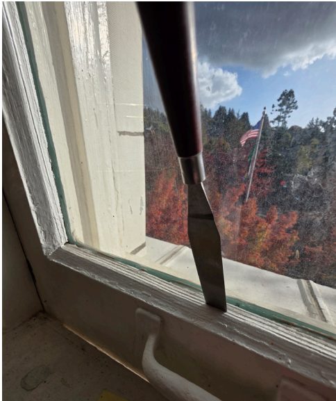
Classroom 19 - South Elevation Recent Paint coatings over 1/2" deep wood rot
