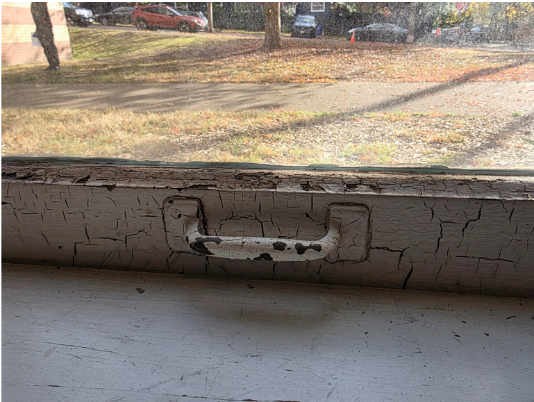
Classroom 2 - South Elevation Paint Failure and extensive wood deterioration. New/refurbishment of hardware required.
