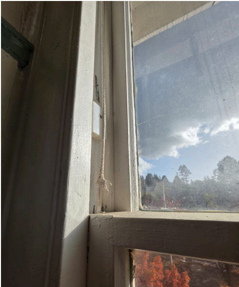
Classroom 19 - South Elevation Recent paint over deteriorating window. Repair sash cord and counterweight.
