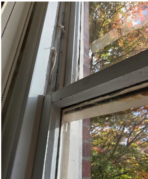
Office 225 - South Elevation Failing paint coating. Sash cord and counterweight need repair.
