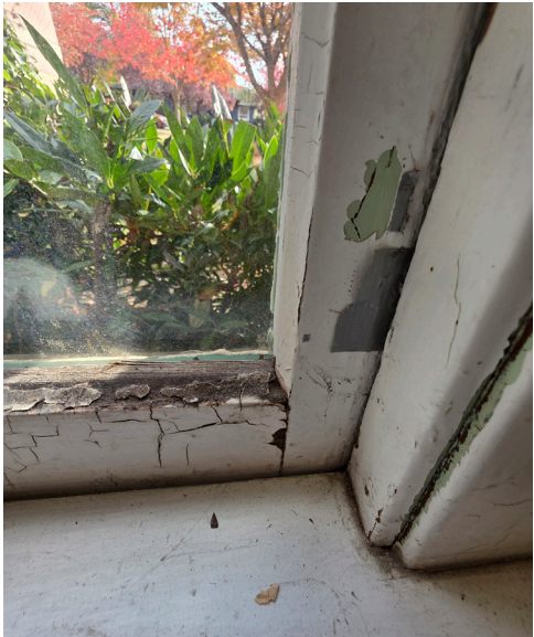
Classroom 2 - South Elevation Window stile is cracked and has been repaired with duct tape.
