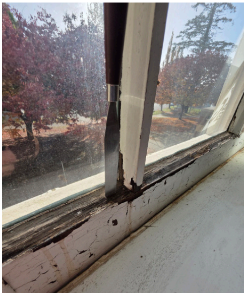
Office 225 - South Elevation Paint Failure and extensive wood Deterioration typical for jambs and bottom rails
