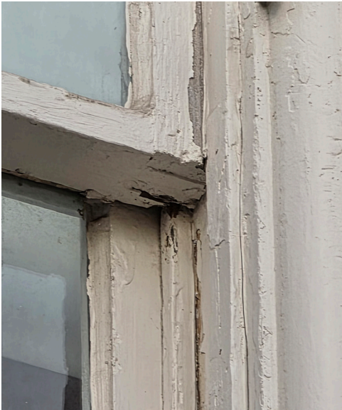
Classroom 1 - South Elevation Paint Failure and extensive wood Deterioration
