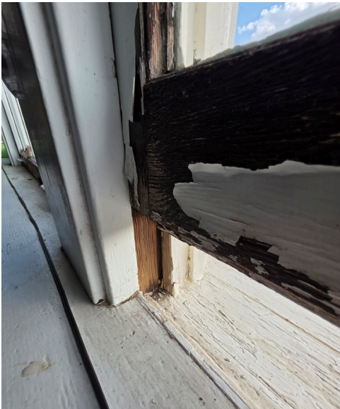
Classroom 17 - South Elevation Parting Bead is failing - this is only window in bay that is still operable.
