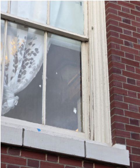
Classroom 9 - South Elevation Paint Failure at exterior
