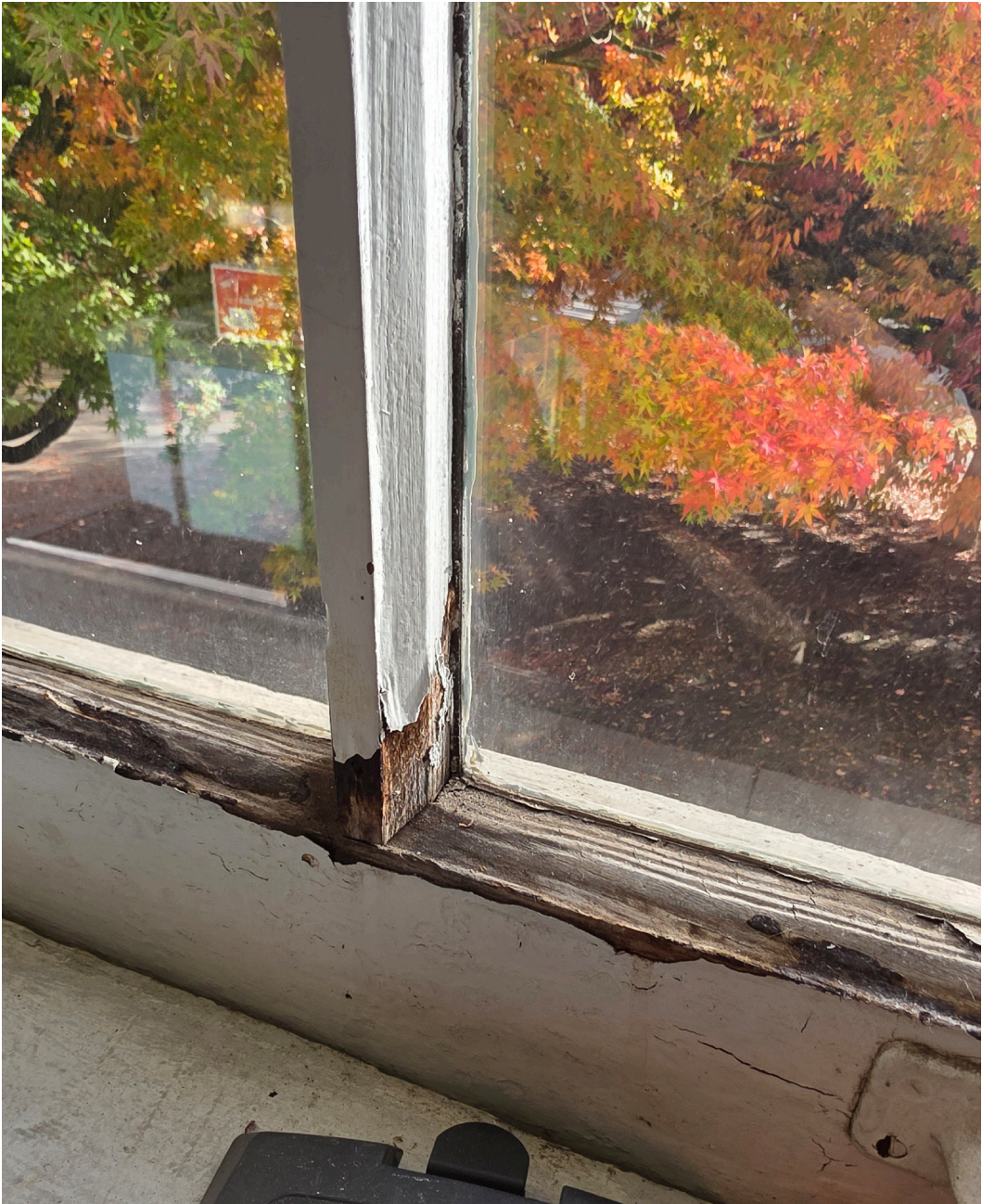
Office 225 - South Elevation Paint Failure and wood deterioration at vertical Muntin to bottom Rail.
