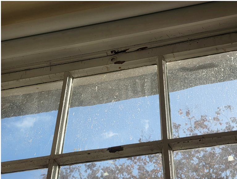
Classroom 2 - South Elevation Paint Failure and extensive wood deterioration at window head. Type-C double hung windows have been secured shut*
