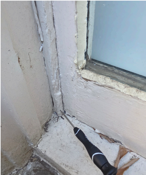
Classroom 1 - South Elevation Paint Failure and extensive wood Deterioration of exterior blind stop.
