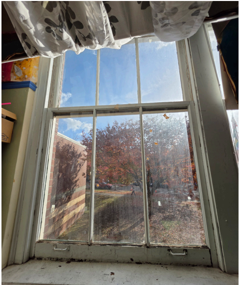
Classroom 9 - South Elevation Complete Paint Failure at interior with areas of wood deterioration
