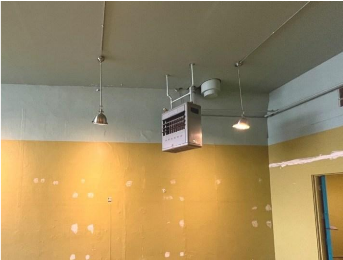
Old ceiling hung Gas Heater.
