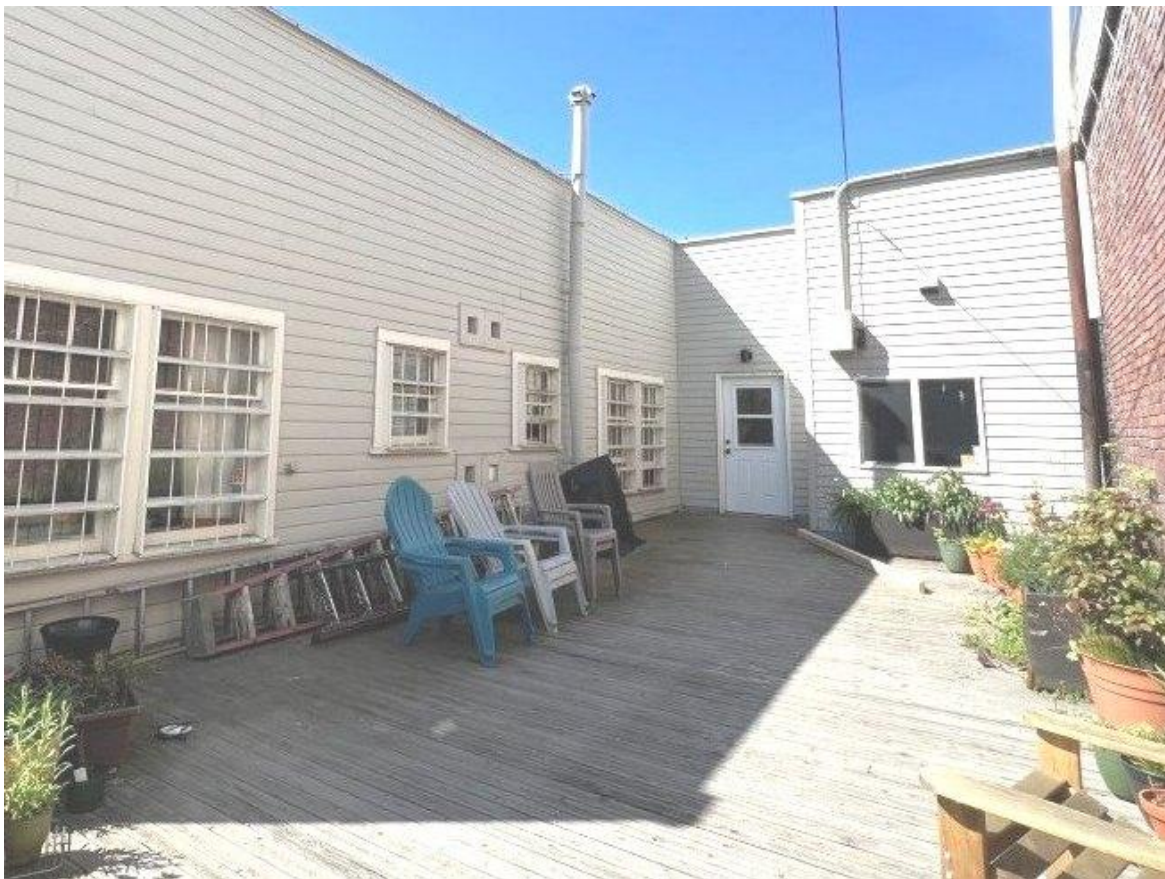
Back Deck with chairs covering broken deck rails.
