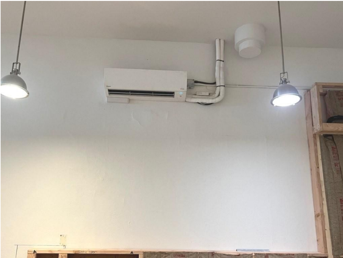
New Electric Heat Pump, providing both cooling and heating.
