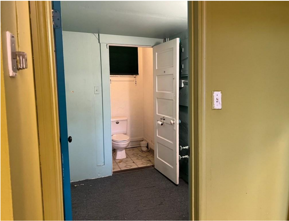
Old non-ADA compliant bathroom.
