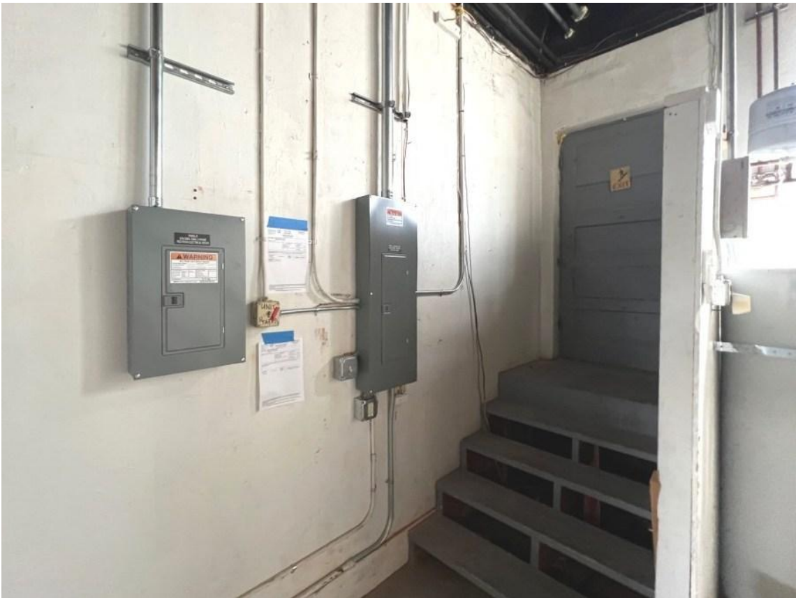
New 200-amp single phase panel and new 100 amp 3-phase panel.
