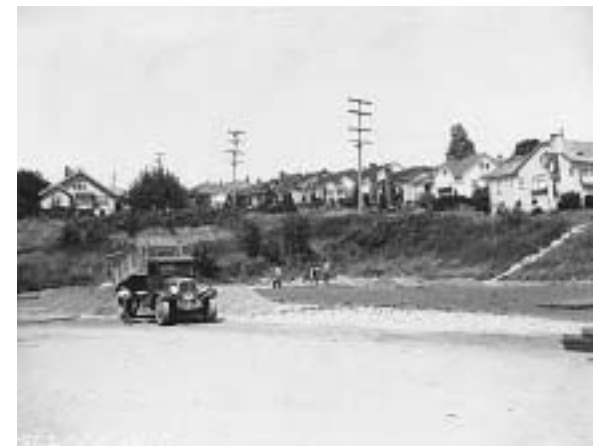
1935 photograph of the former Franklin High School tennis courts during construction. Source: University of Washington Libraries, Special Collections, UW207952.
