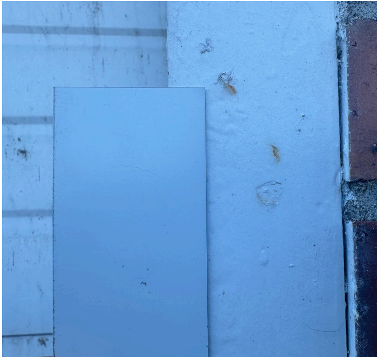
at location of proposed door replacement
