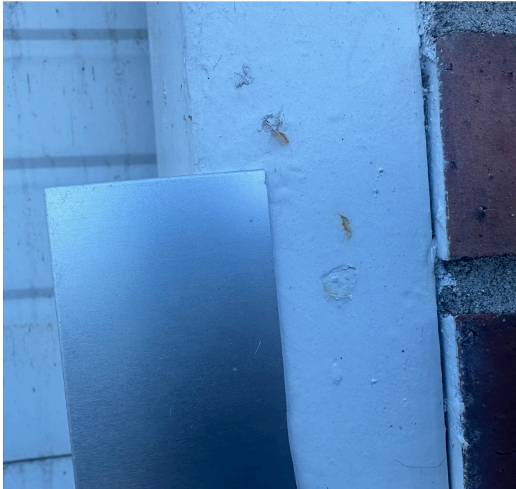
at location of proposed door replacement
