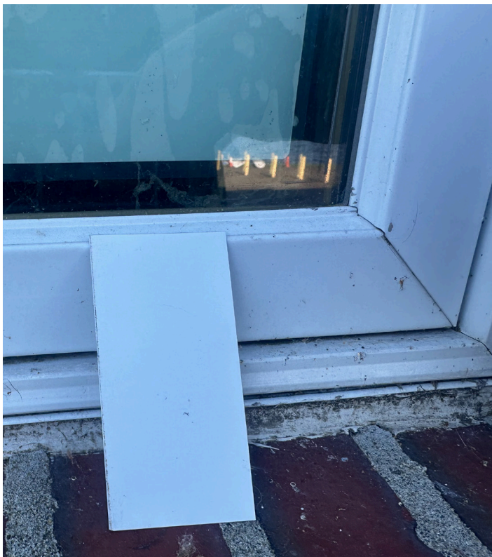
in proximity to other materials on building
