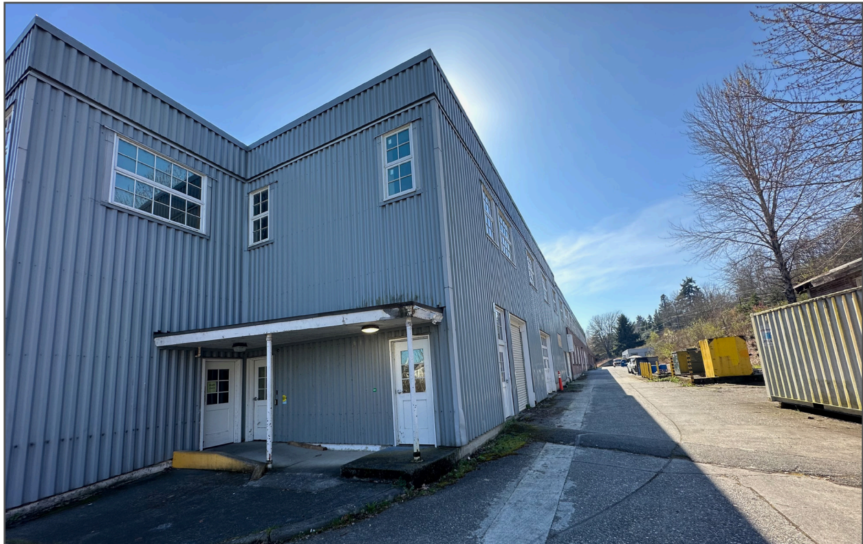
Figure 16 • western end of northern facade viewing south down western facade at alley
