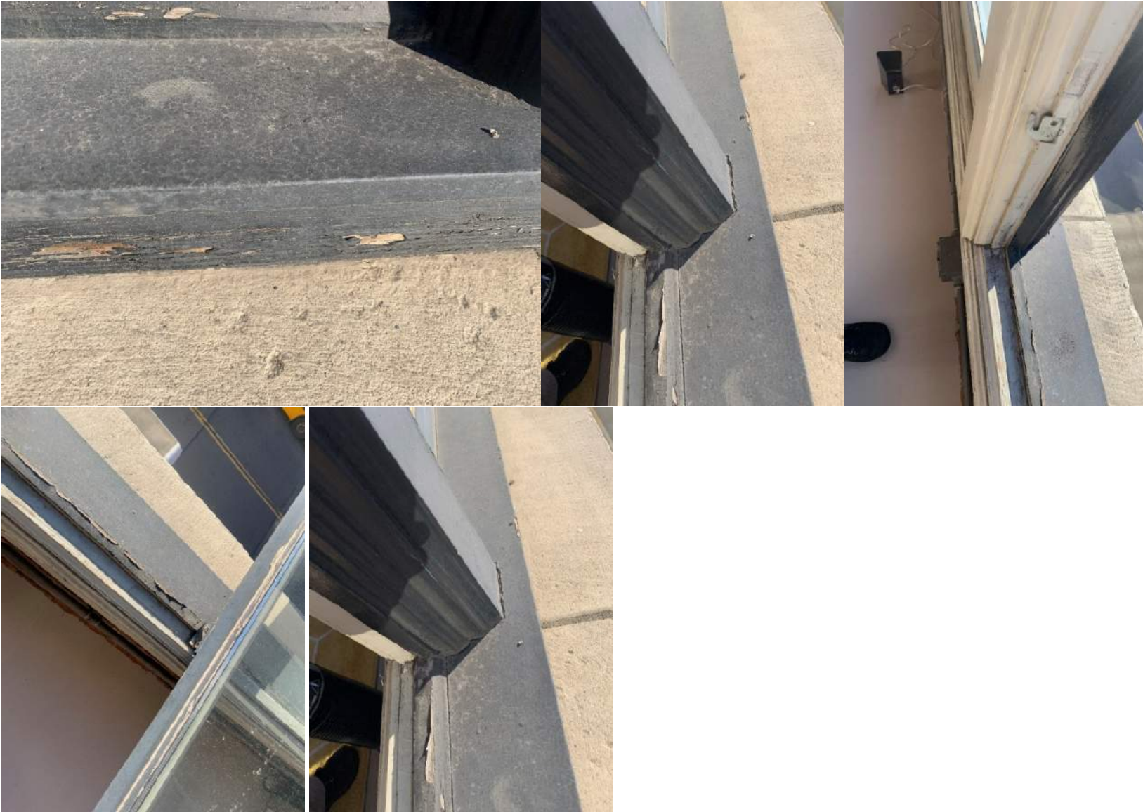
Unit 3A – Upper row (L) weatherchecking at sill. (C) weatherchecking and peeling paint at sill. (R) peeling paint and damage at frame and sill.
