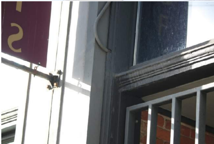
South (212) : Upper Left – staining and related damage at upper sash / muntin’s. Upper Right – weathered brick at jamb and sill trim Lower Left – intersection of brick mold at jamb and horizontal mullion showing weathering .
