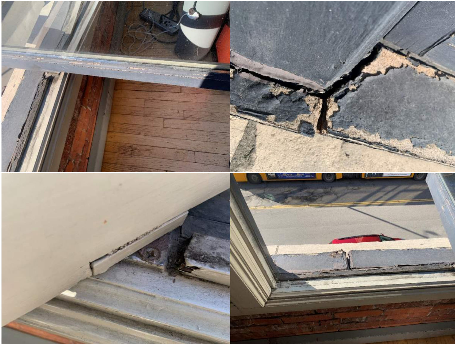
Unit 2C: Upper photos – (L) Damage at sill and sash. (R) Damage to frame, and sash. Lower photos – (L) Damage at pivot hardware, Right damage at sill and frame.
