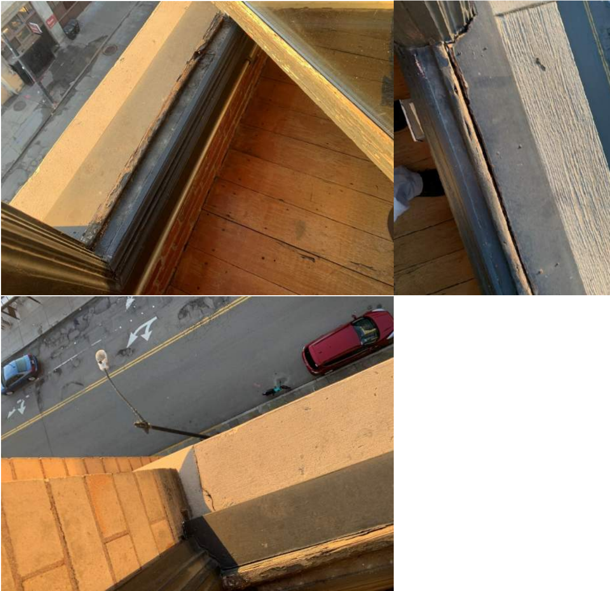
Unit 5C: photos showing checking and rot in sash and glazing stops particularly near the sill.
