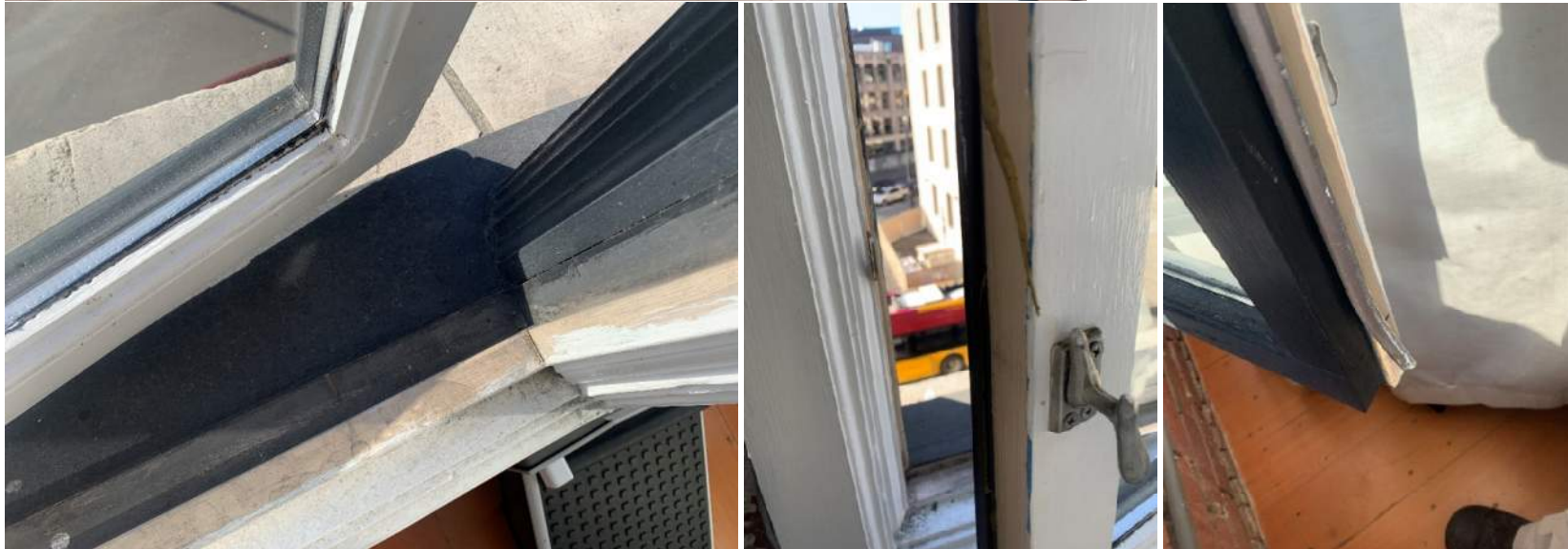
Unit 3C: Lower row – (L) open joints and paint damage, (C) paint damage (R) damage to weatherstripping.
