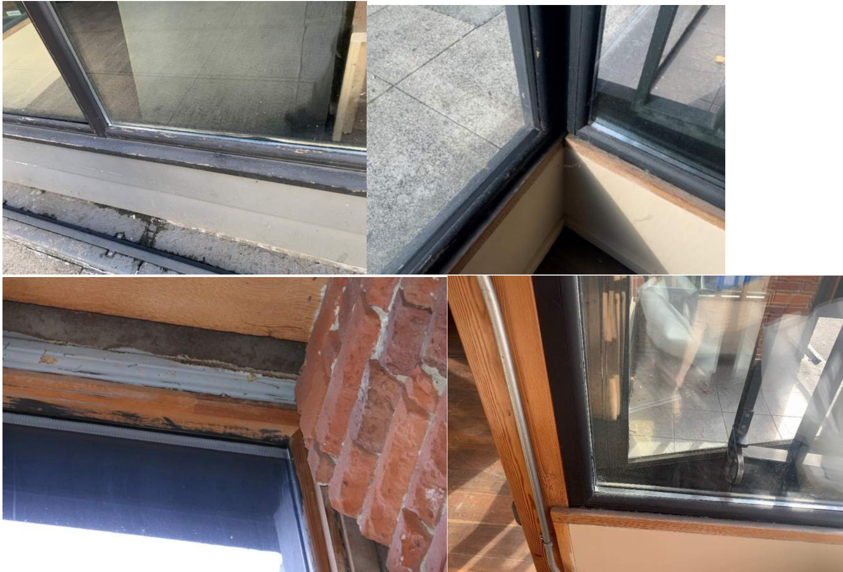
North Storefront (208-210): Upper Left Photo - Weatherchecking and environmental damage at sill. Upper and lower right photos - weather checking at interior of storefront in unit 208.
