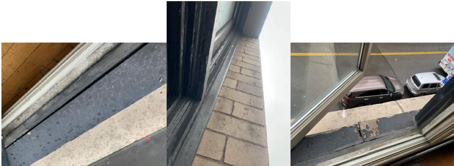
Unit 2A: (L) damaged to sill and exterior of window frame. (C) Exterior wear at jamb. (R) Damage to sill trim.
