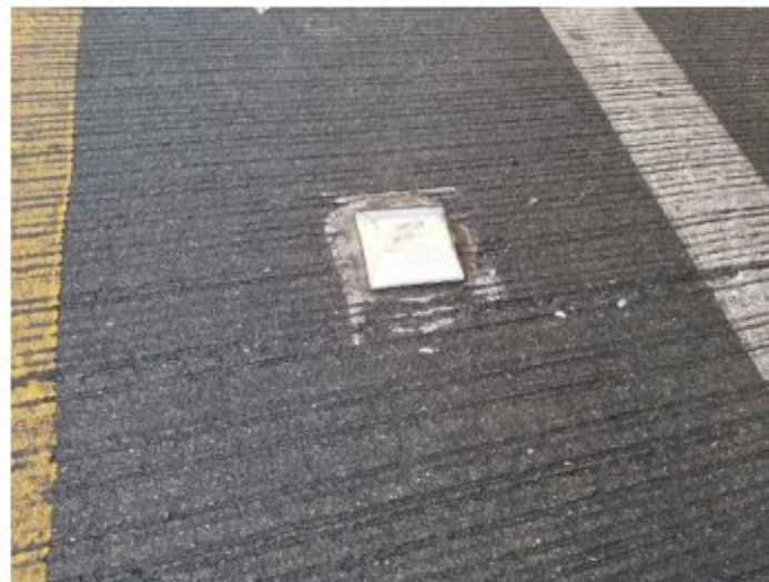
Reflective Pavement Mark
