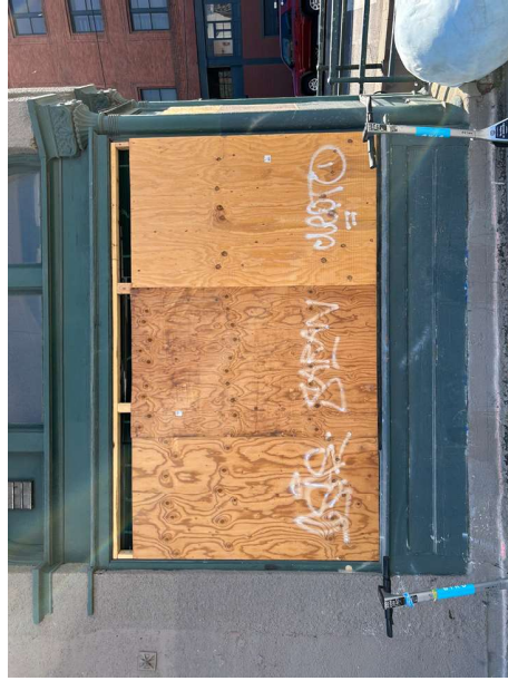
2. DAMAGED AND ROTTING STOREFRONT AT WEST ELEVATION
