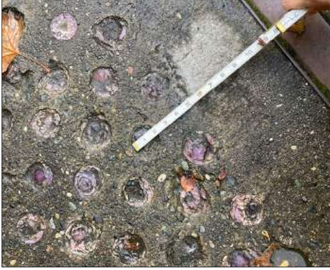
Figure 13 – Zoomed in view of the existing and deteriorated round glass pavers within the red outlined area in figure 11. The diameter is 2 inches. (Source: Seattle City Light, 2023.)
