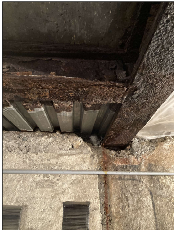
Photo 7 – Detail view showing general conditions of the steel beams and ceiling decking in the vault. (Source: SCL, 2022.)
