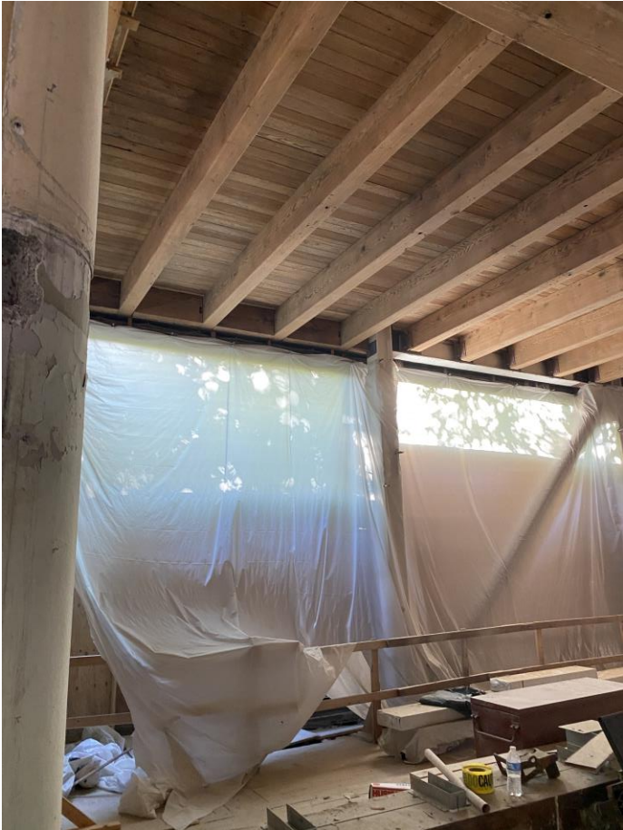
September 2021 – Exterior Penetration
