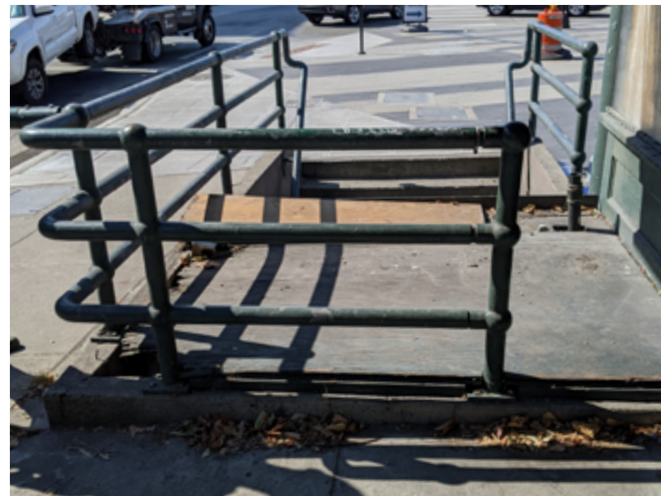
DAMAGED VENDOR PLATFORM OVER STAIR
