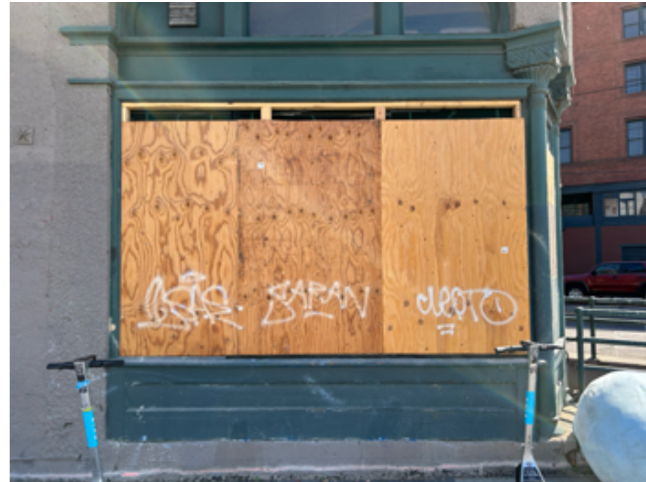
DAMAGED AND ROTTING STOREFRONT AT WEST ELEVATION
