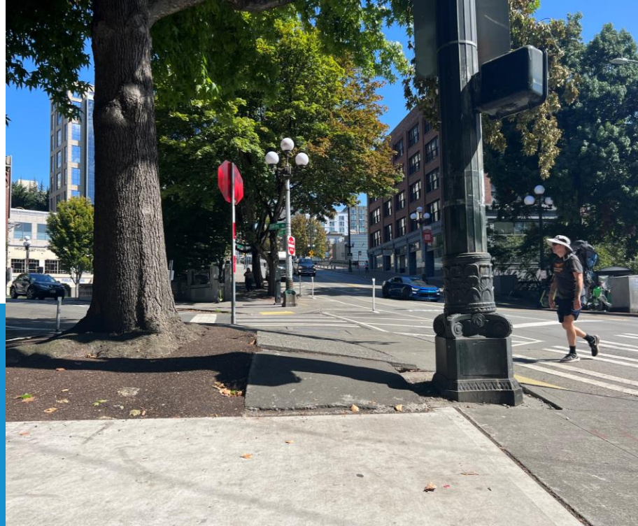
Heaved sidewalk at City Hall Park
