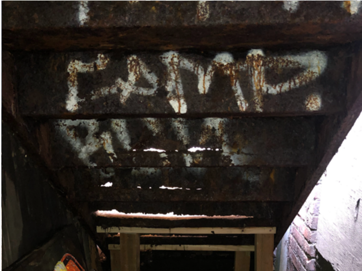
FROM BELOW STAIR SHOWING LEVEL OF DETERIORATION
