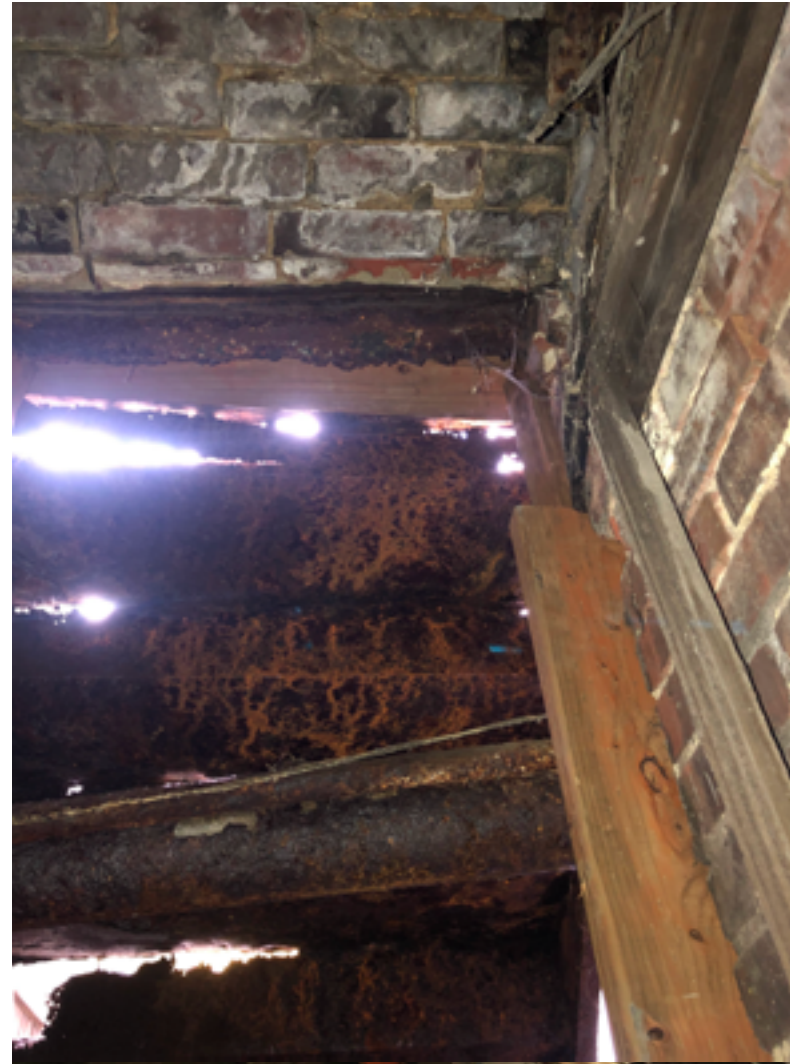
FROM BELOW STAIR SHOWING LEVEL OF DETERIORATION
