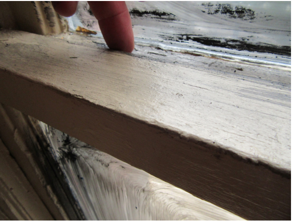
POOR cord & misaligned
