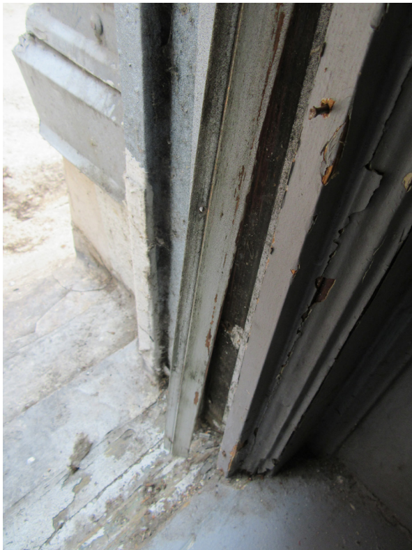
POOR Sill & Frame
