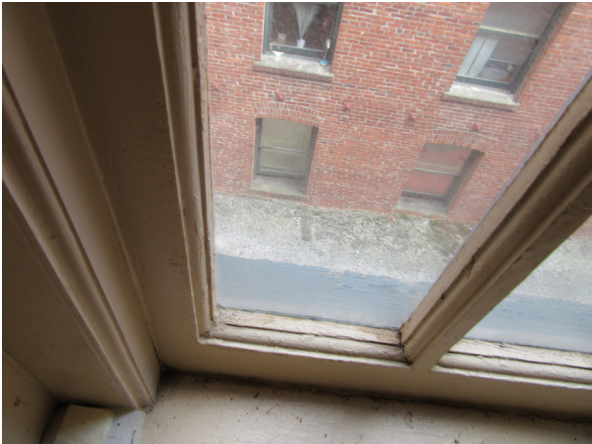
POOR Sill FAIR Single Glazing
