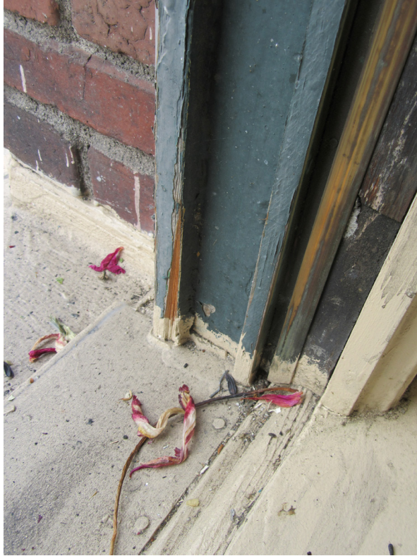
POOR Frame & Sill
