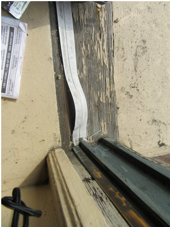
POOR W.Stripping & Frame
