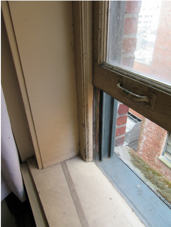
FAIR Sill, Frame, W. Stripping, Stool, Trim POOR Sash
