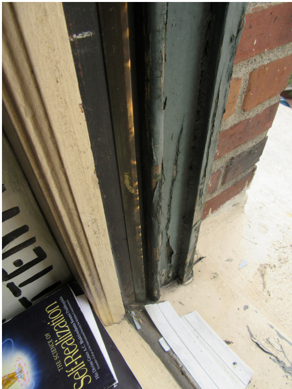
POOR Frame & Sill
