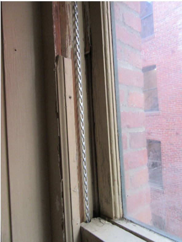
POOR Frame and W. Stripping
