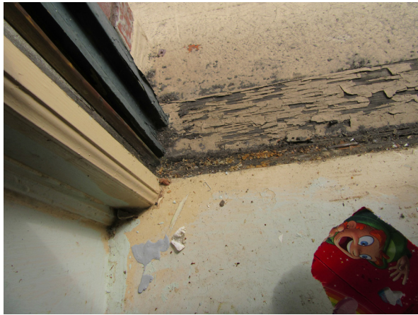
POOR Sill & Frame
