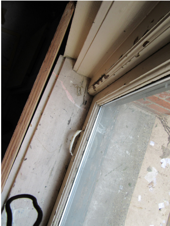
POOR Frame & Sill
